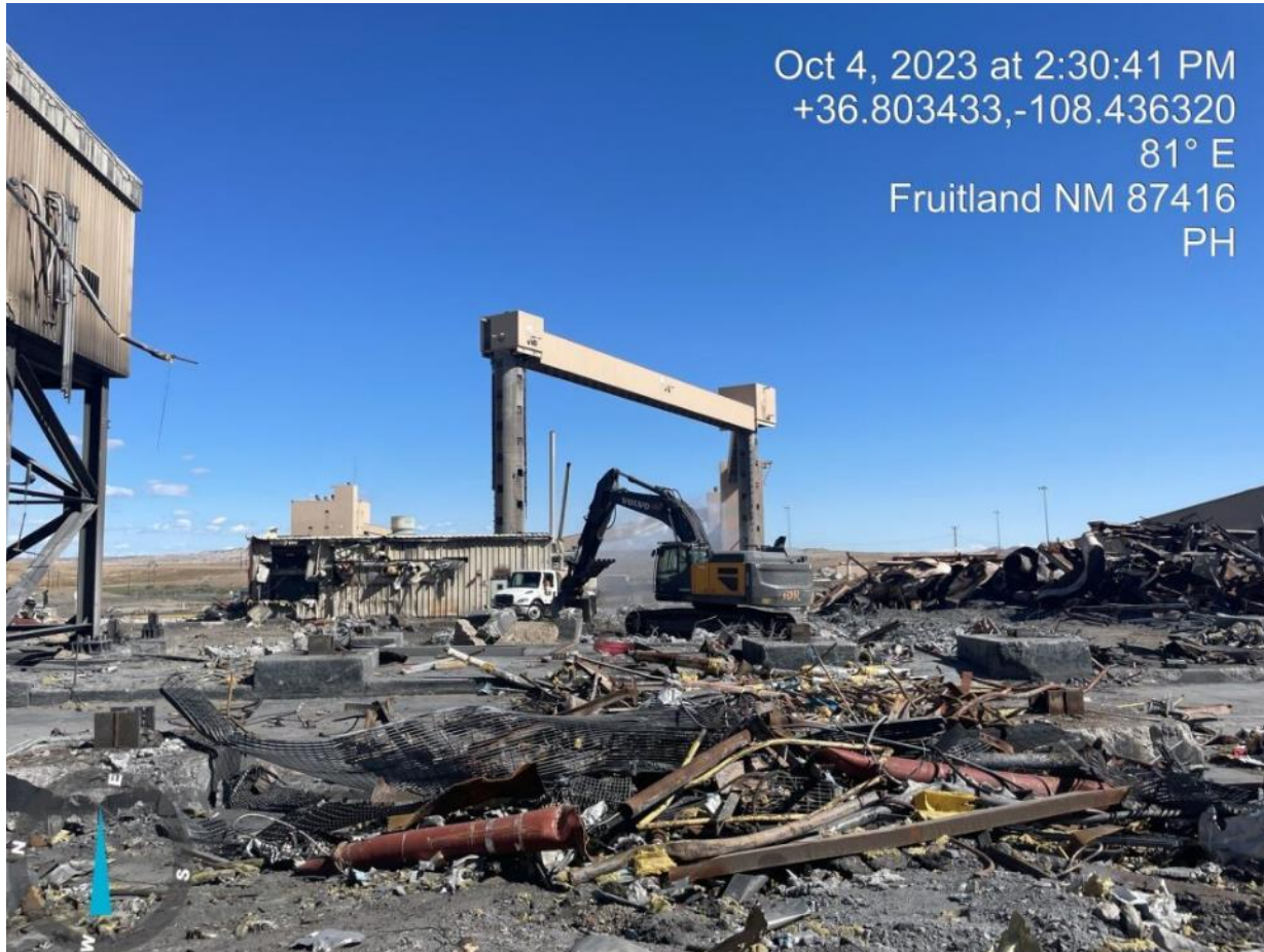
Grizzlies (coal conveyors)
