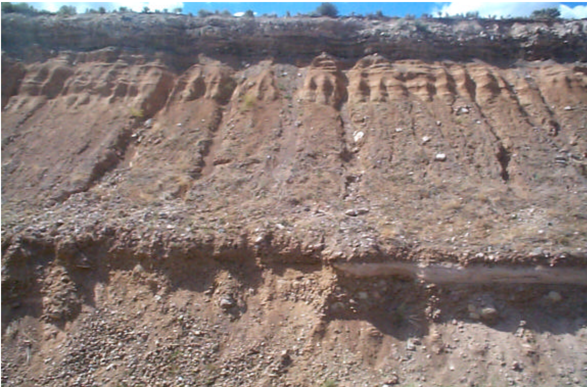
Photo 28: Moderate gullies in the west slope of the West Diversion Ditch at survey stop D-1.
