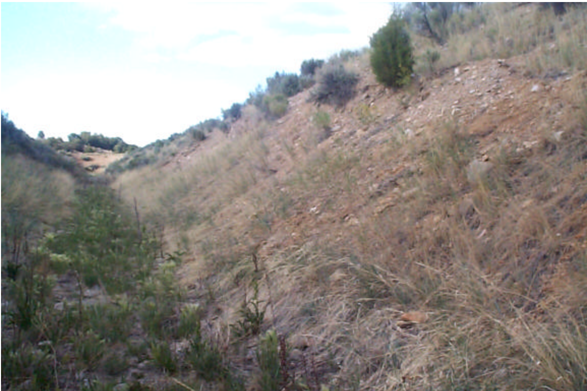
Photo 22: Looking north at the east slope of the East Diversion Ditch from survey stop E-6.
