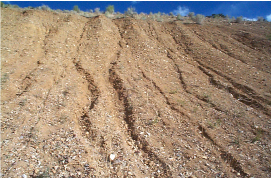
Photo 26: Small to moderate gullies in the east/south slope of the East Diversion Ditch at survey stop E-14.
