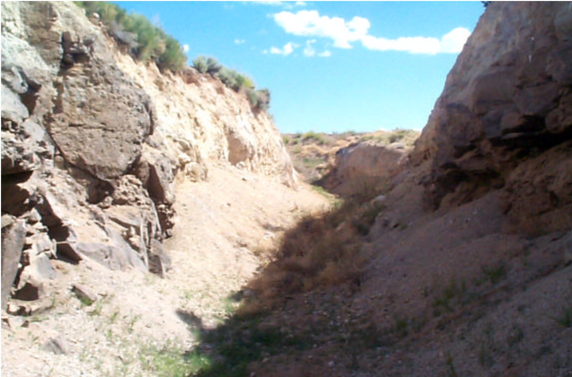
Photo 31: West Diversion Ditch looking south near survey stop D-5 (near vertical side-slopes).
