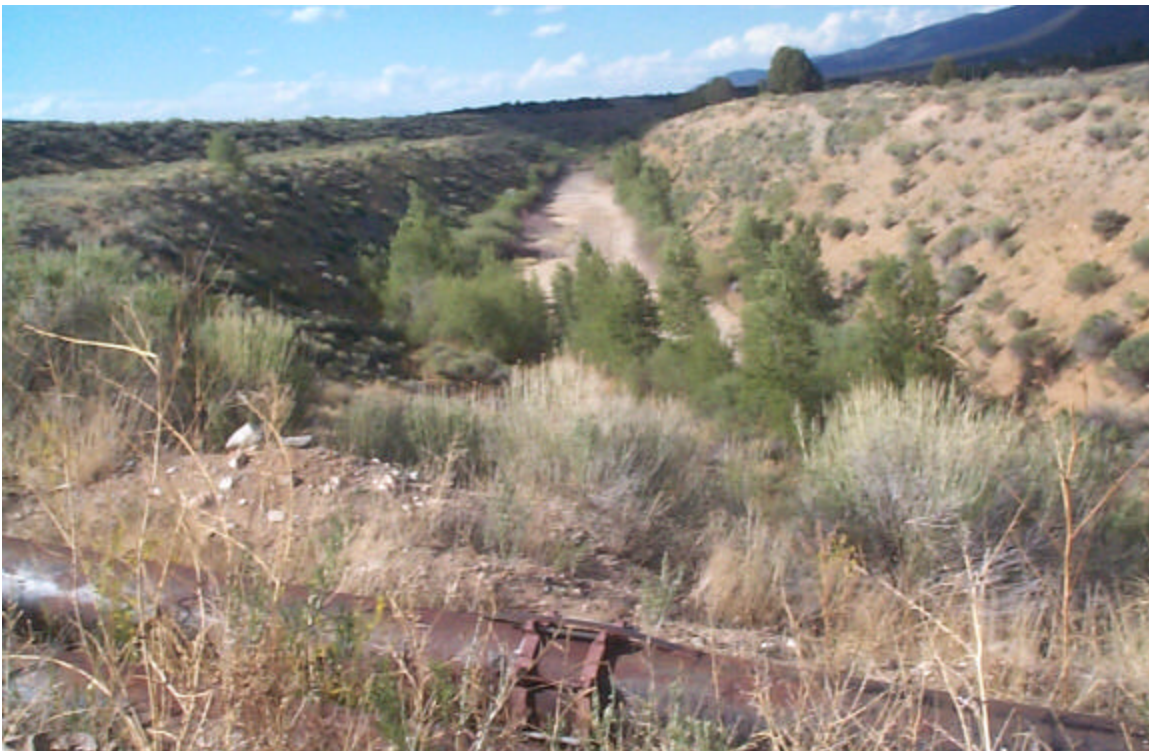
Photo 20: East Diversion Ditch looking north from the road crossing at survey stop E-4.
