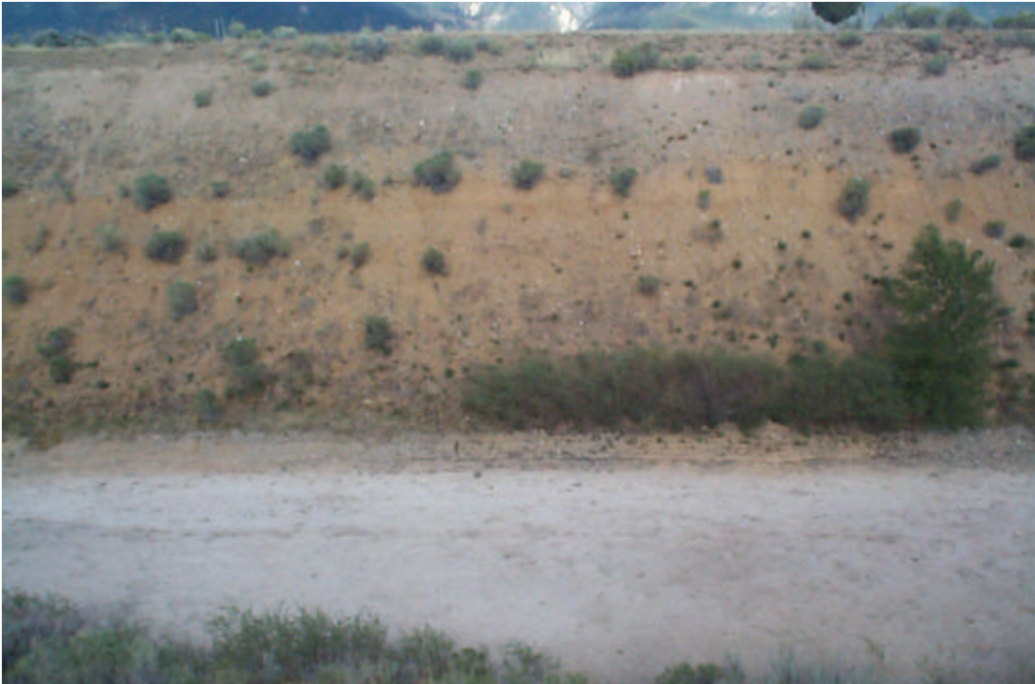
Photo 19: East slope of the East Diversion Ditch at survey stop E-3 (no erosion; dry channel bottom).
