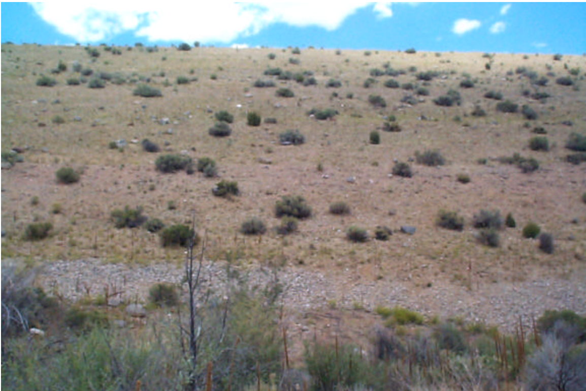
Photo 8: Middle section of the downstream face of Dam 4; coarse rock layer at the toe.
