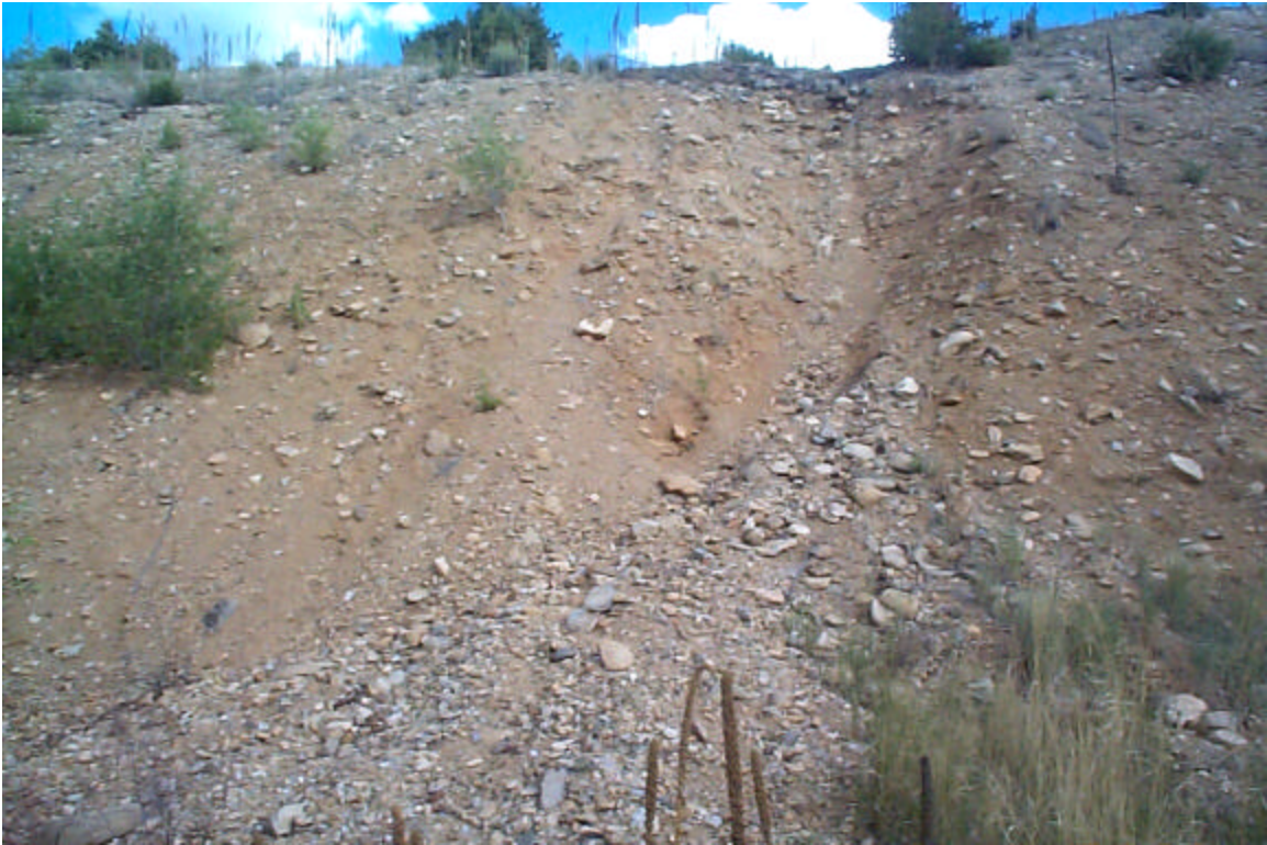
Photo 23: Small gully in the east slope of the East Diversion Ditch at survey stop E-7.
