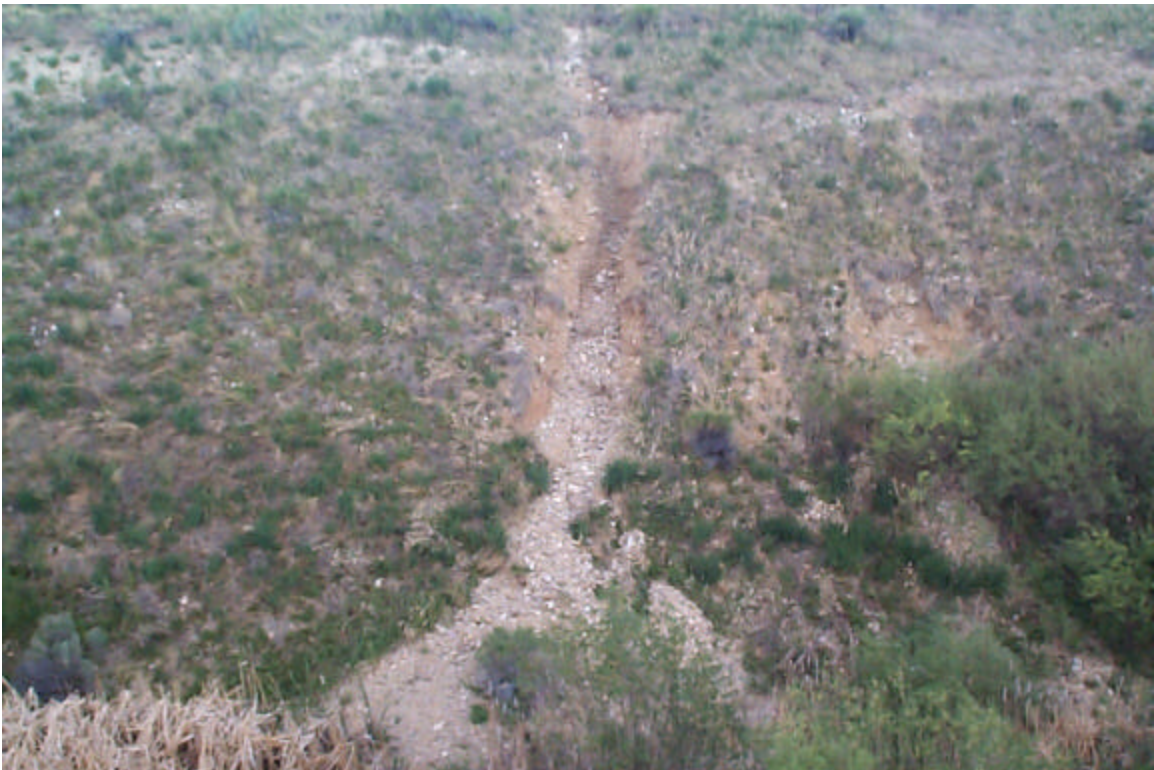
Photo 18: Small gully in the east slope of the East Diversion Ditch at survey stop E-2.
