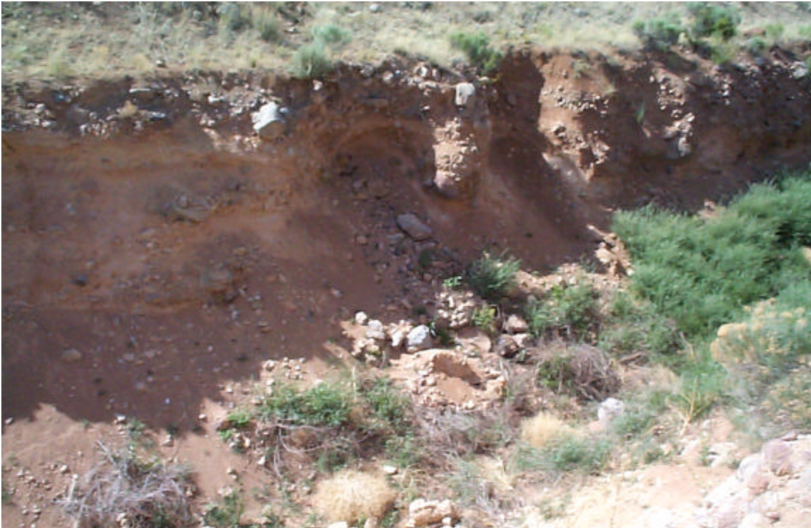
Photo 29: Cave-ins on the west slope of the West Diversion Ditch and fallen debris in the channel bottom at survey stop D-2.
