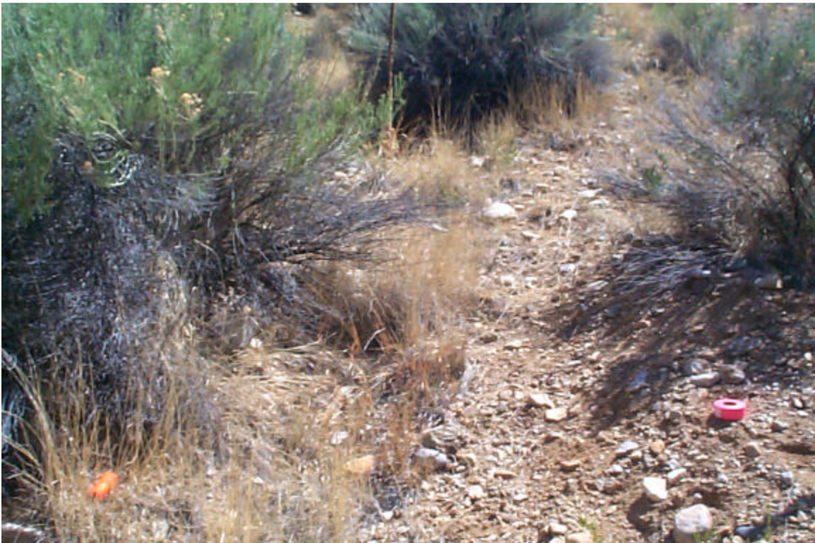
Photo 6: Small gully near the toe of Dam 1; pink flagging tape at the edge of the gully.
