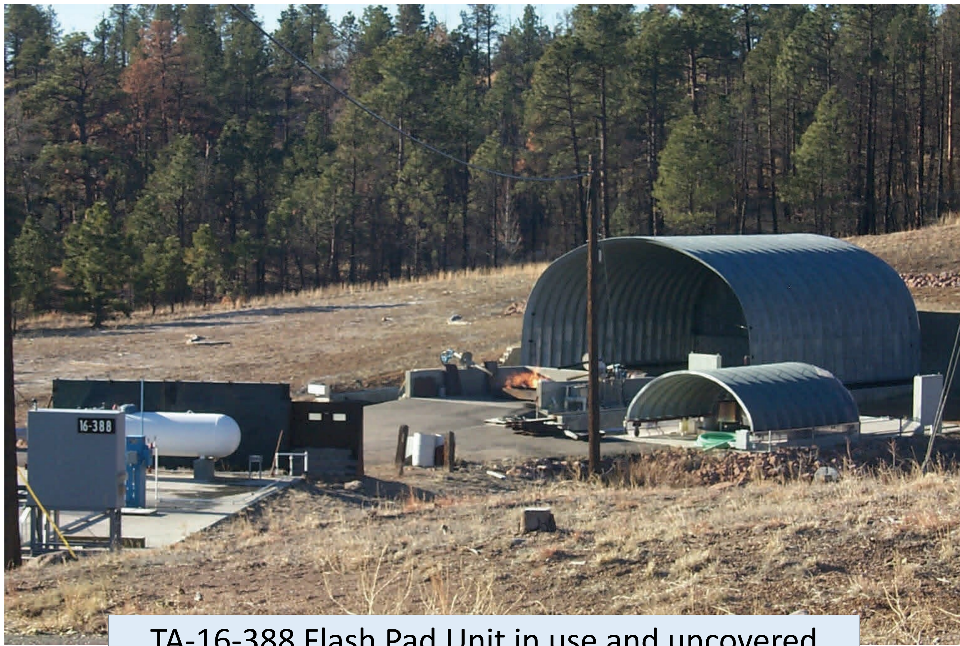
TA-16-388 Flash Pad Unit in use and uncovered
