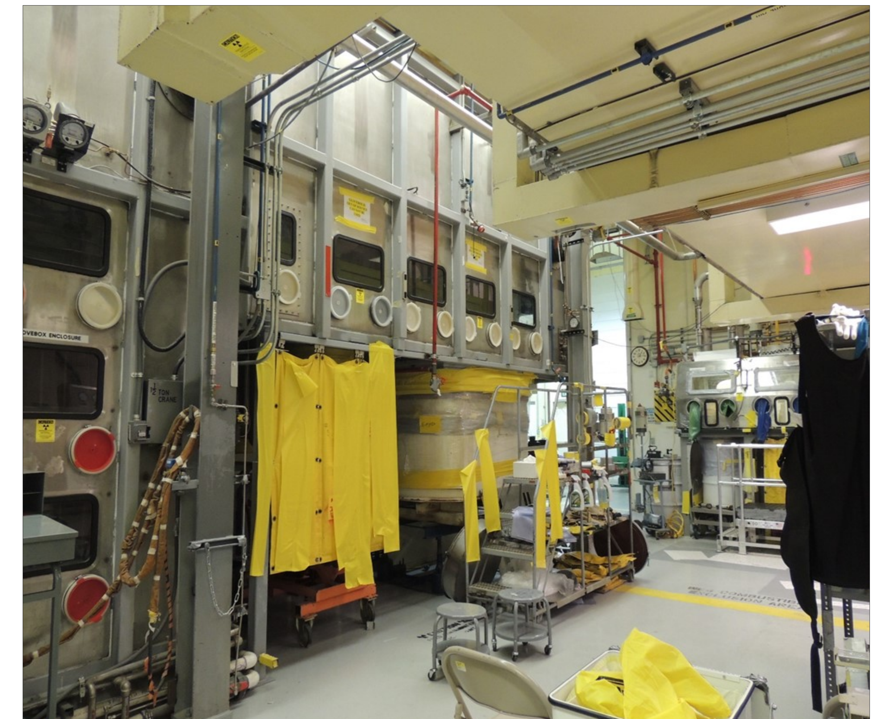
TA-50-69 Indoor, Rooms 102 and 103, Waste Characterization, Reduction, and Repackaging Facility (WCRRF)
