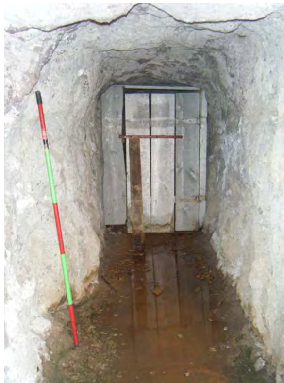
Photo 23-Looking south at Adit-2 in the Western Area. Photo is similar to photo in Anderson Report.
