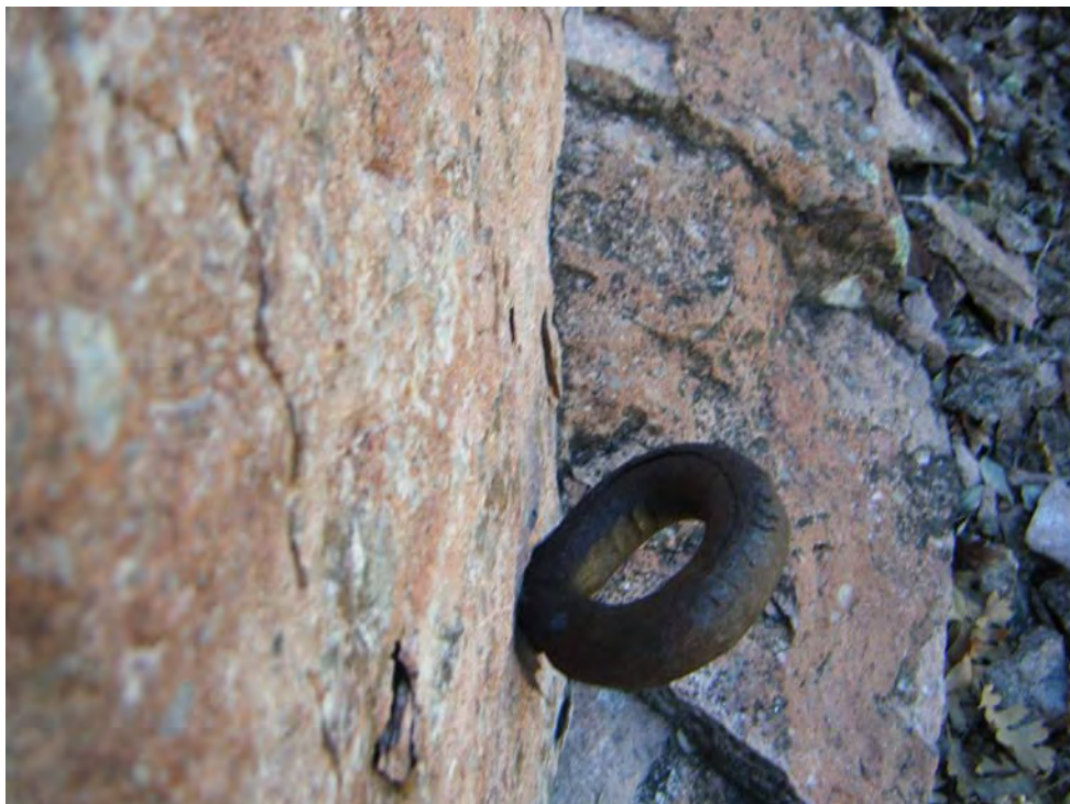
Photo 4-Looking west at an eyebolt (Equip-1) attached to the rock face in the Eastern Area.
