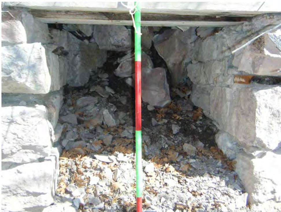
Photo 10-Looking at a collapsed hole in StrucLn-1 in the Eastern Area.
