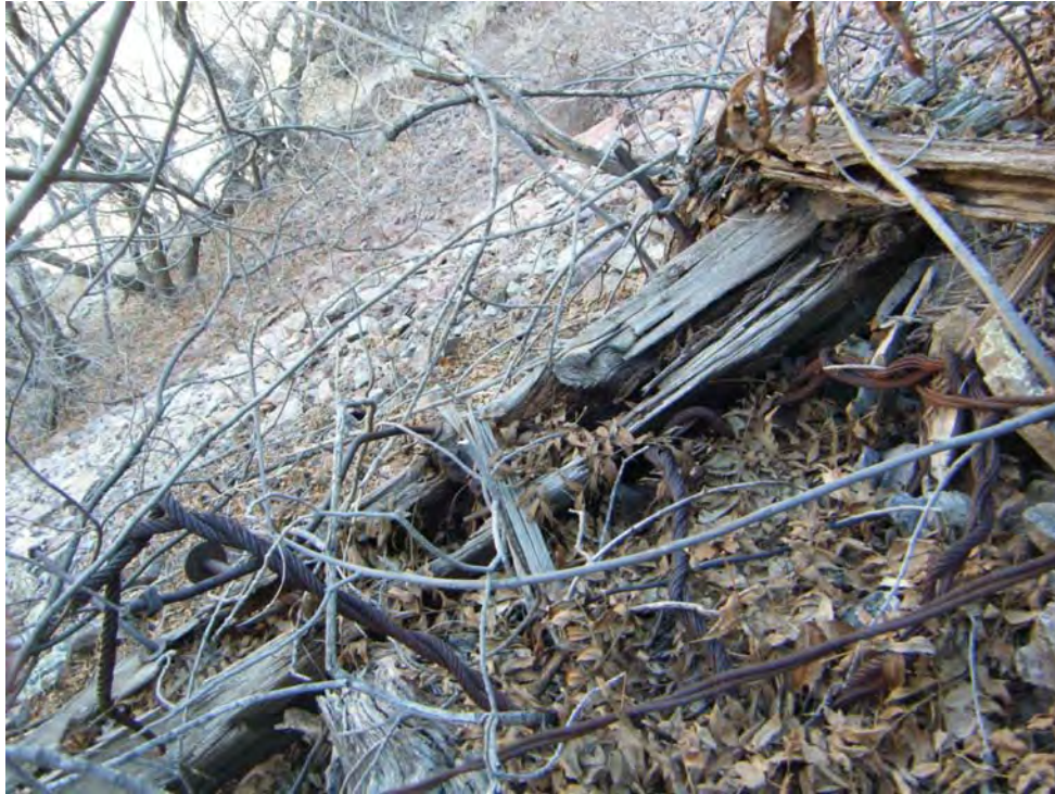
Photo 3-Looking north, down slope at wooden beams and cables in the Eastern Area.
