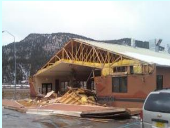
Winds damaged the Elderly Day Care Center at Mescalero NM . (Mereya Braden Ruidoso News)
