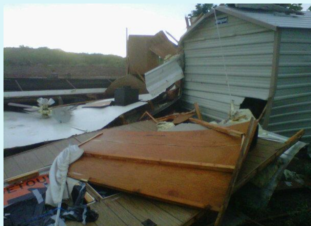
Gila NM property damage. (Loretta Brown)
