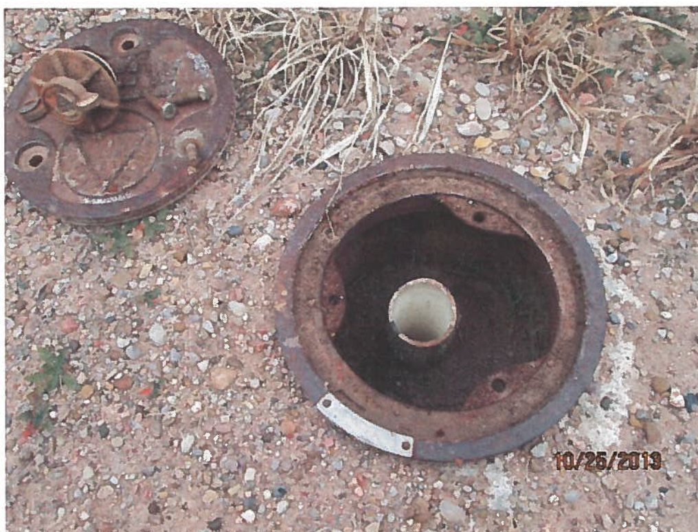
Photograph 3. MW-2A casing and well cover, both in relatively good condition.
