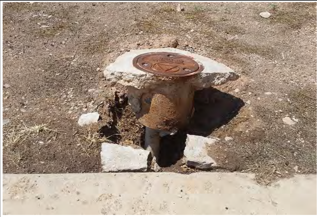
1. Damaged monitor well MW-3 surface completion.
