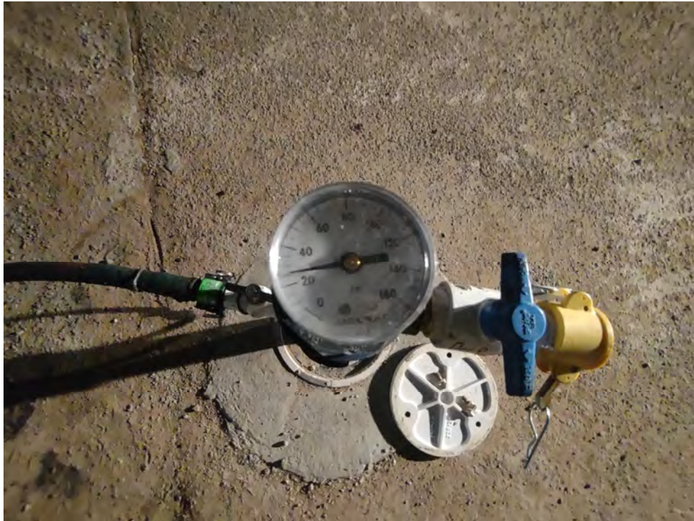
Wellhead Assembly – View from Above
