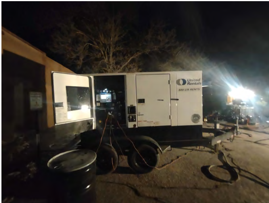
Trailer-Mounted MultiQuip 150 KVA Generator
