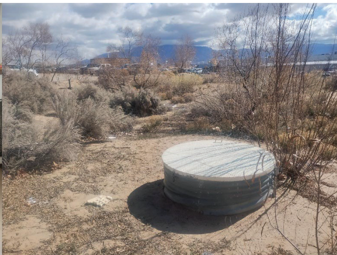
CW-2 Well vault
