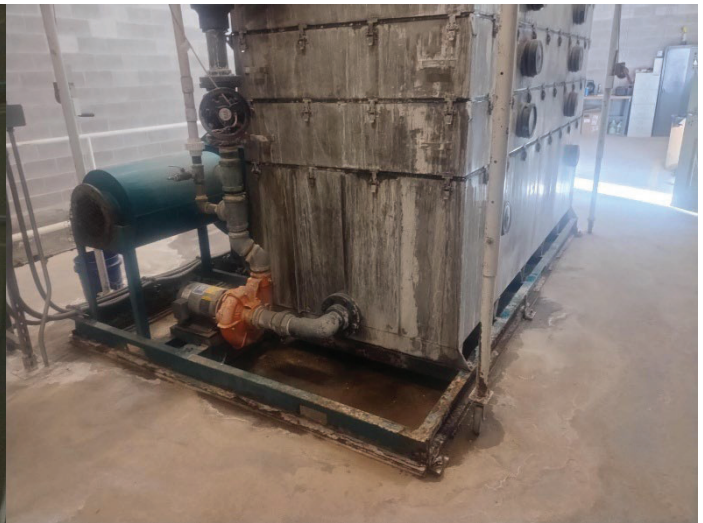
CW-1 Air Stripper
