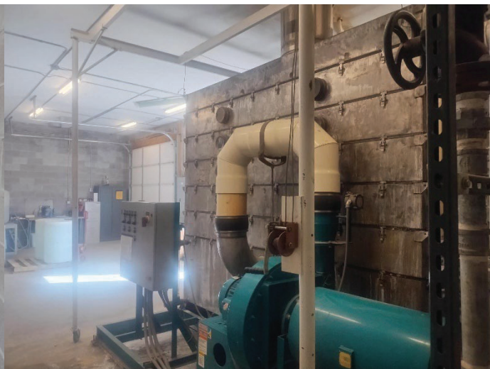
CW-1 Air Stripper
