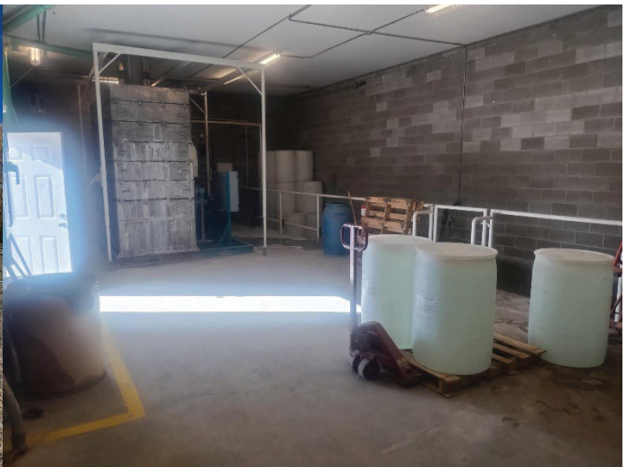
CW-1 Pump house interior with aquamag drums
