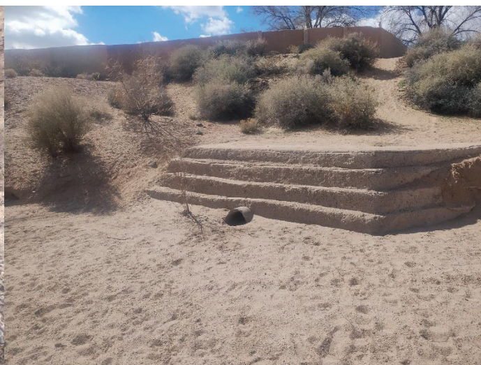
CW-1 Infiltration Gallery Looking South
