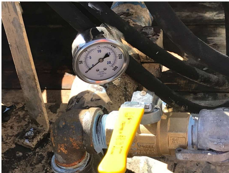
Injection Pump, Pressure Gauge, and Shut-Off Valve
