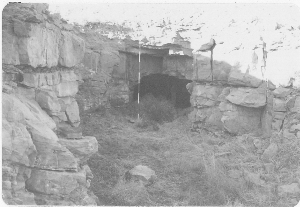
Photo (d) Close-up of adit shown at end of trench in photo (c). Portal is 5' x 6', workings go in about 22'. Note range pole for scale.
