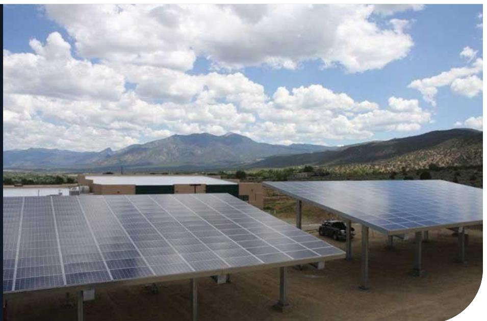
Solar arrays similar to those installed at the Taos Wastewater Treatment Plant
