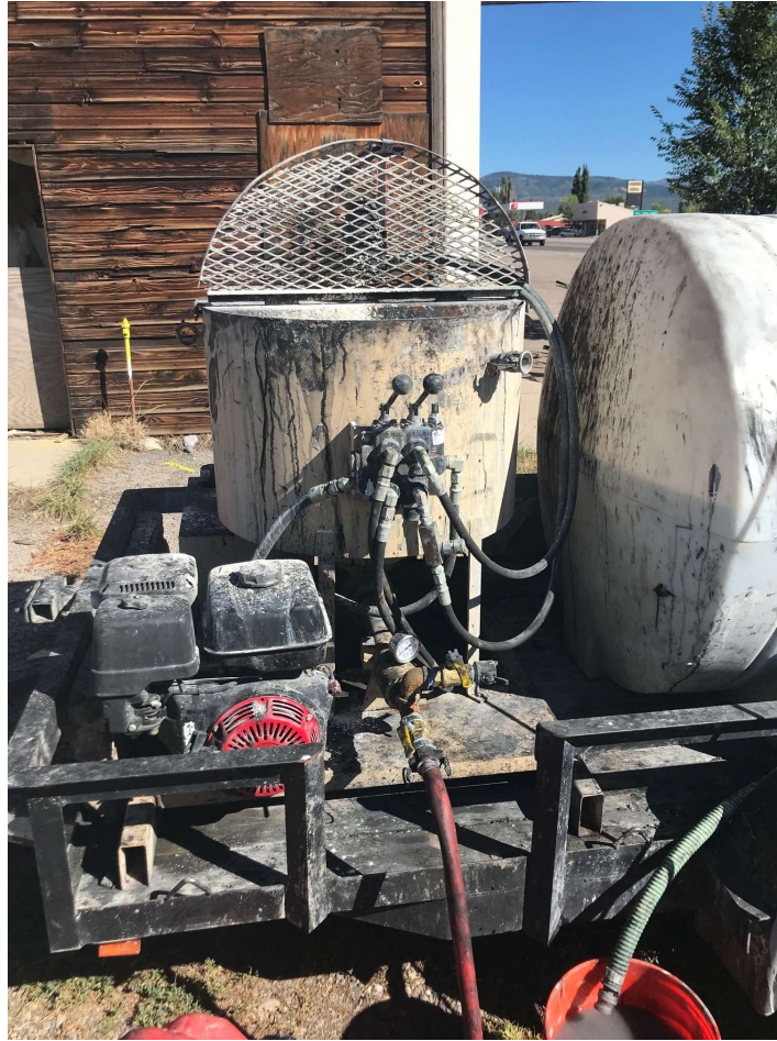
Mixing Vessel, Pump, Pressure Gauge, Generator
