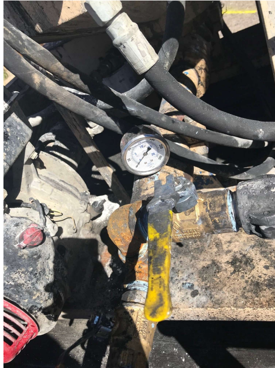
Injection Pump, Pressure Gauge, and Control Valve
