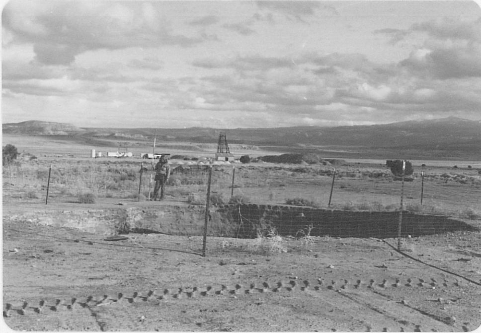
Photo (a) View eastward of caved mine shaft at Isabella Mine; Spencer Shaft is visible in background.
