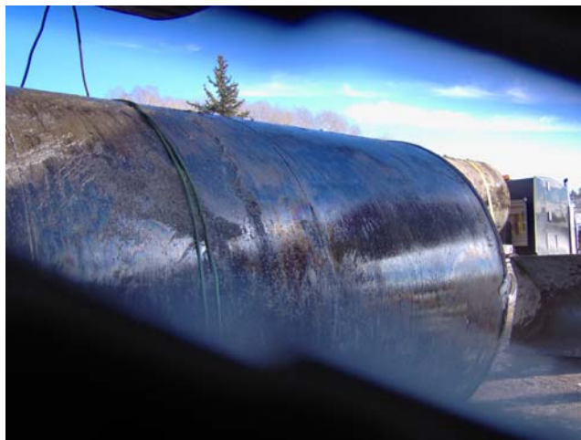
Photo 21: Sheen on UST.
