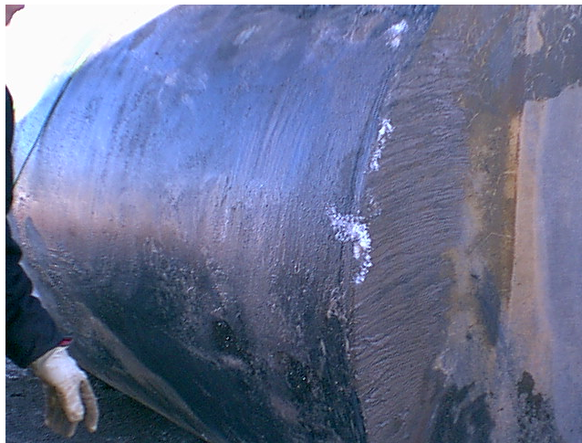
Photo 9: Sheen on UST.
