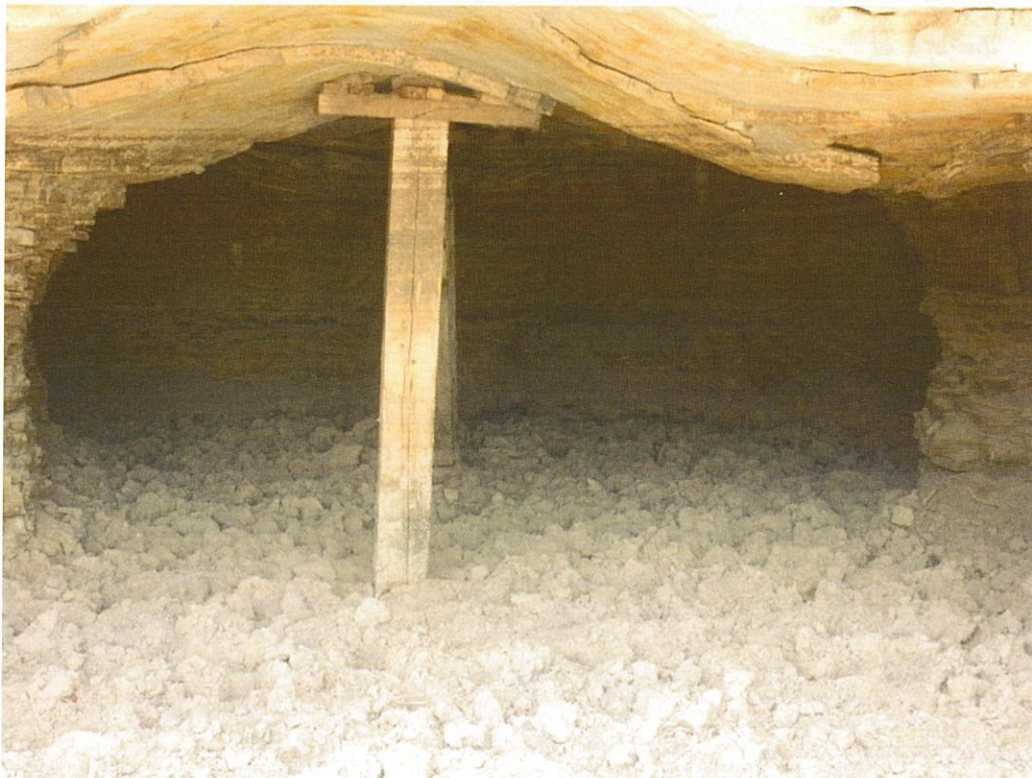
Wooden beam supporting the adit. Evidence of past pooling water as hoof prints were left behind in the now dried mud. Photo taken March 2011, by LaDonna Turner, EPA R6.
