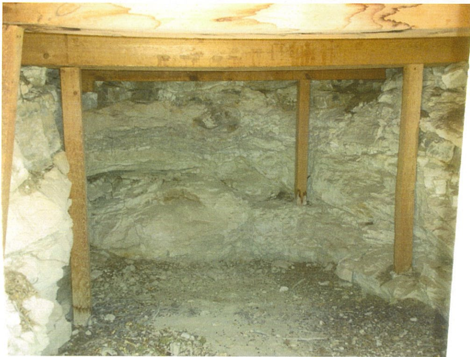
Interior of the dugout. Photo taken March 2011, by LaDonna Turner, EPA R6.
