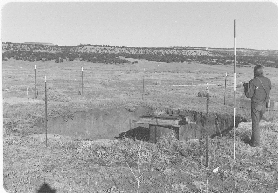
Photo (d) Caved ventilation shaft just west of metal shed shown in photo (a).
