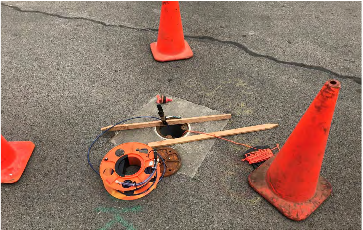
Photo 3: Monitoring well MW-27 with slug and transducer installed in well.
