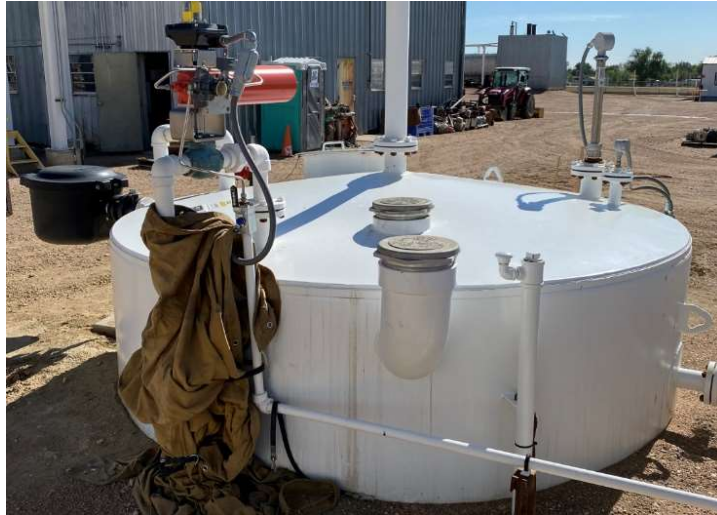
Figure 2. Example of stand-alone condensate tank at a compressor station
