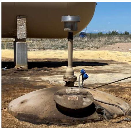
Figure 1. Example of condensate storage tank that would need replacement under new rules.
