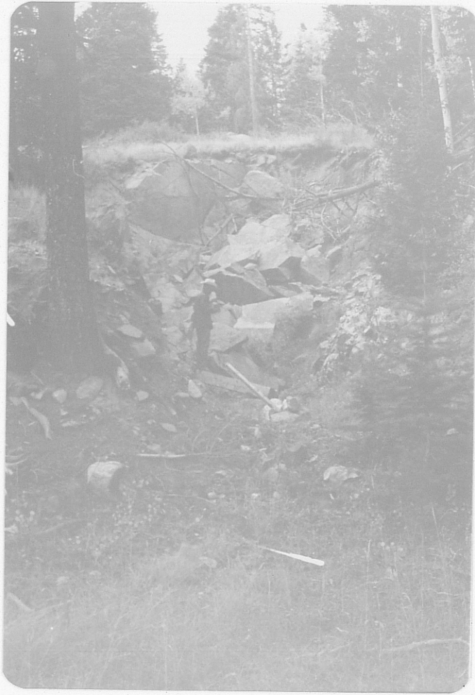
Photo (b) Collapsed workings J.O.L.
