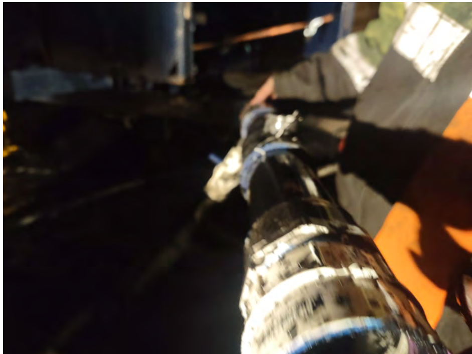
DV-4 Fitting Blew Off of the Wellhead
