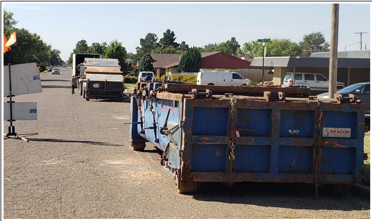
38. Delivery of an empty mud box with a full one awaiting removal (view to south)
