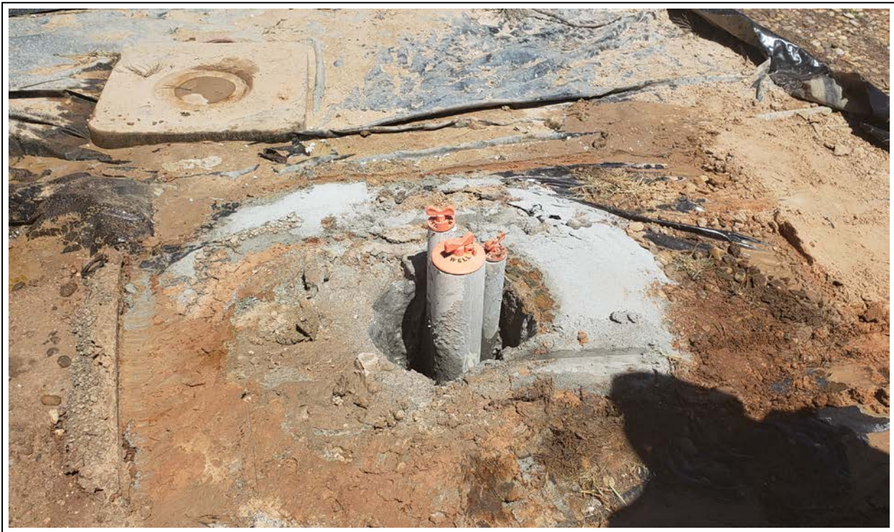
20. RW-1 shallow, intermediate, and deep wells installed before vault completion (view to northwest)
