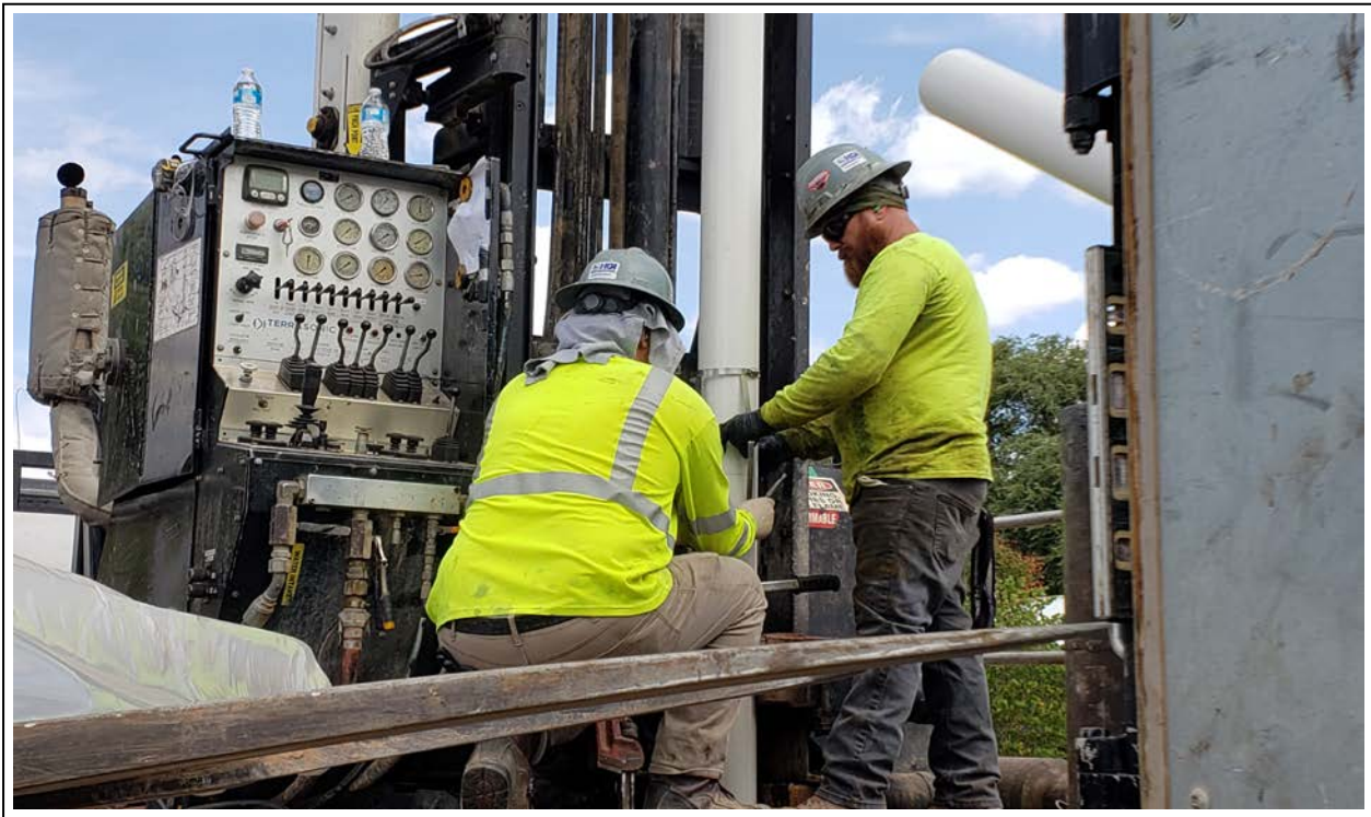
40. Attaching a centralizer to the 5-inch well casing for MW-14 (view to southwest)
