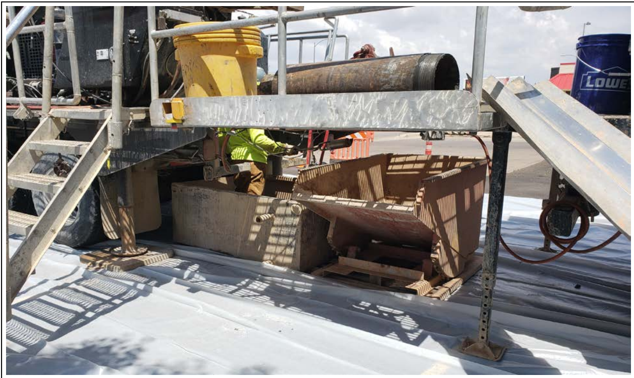
30. Utility clearance with a hand-auger prior to drilling at MW-13 (view to north)
