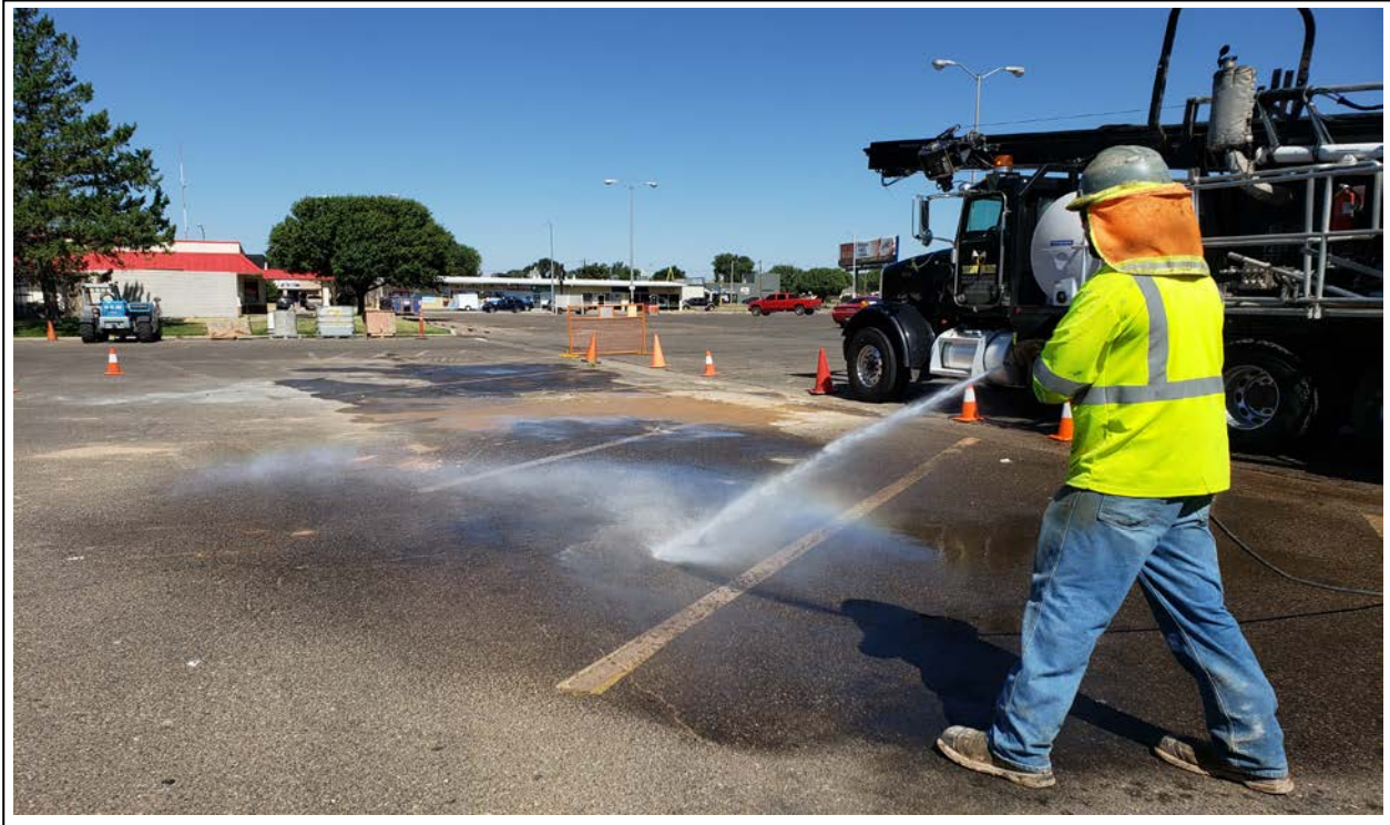
23. Power washing the parking area following drilling at MW-12 (view to west)
