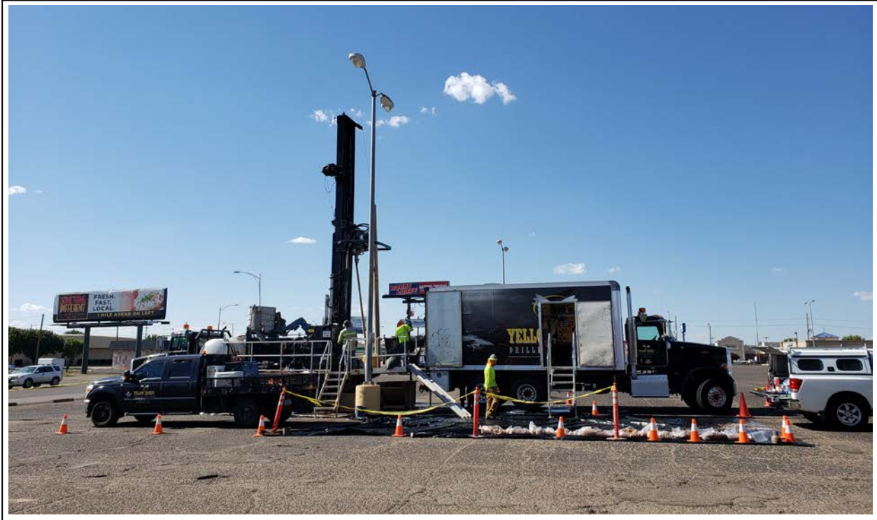
25. Rig and box truck set up for drilling at BW-7R (view to north)
