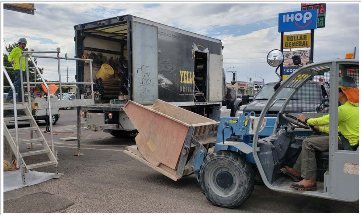
32. Placement of the hopper to contain cuttings from RW-3 (view to northwest)
