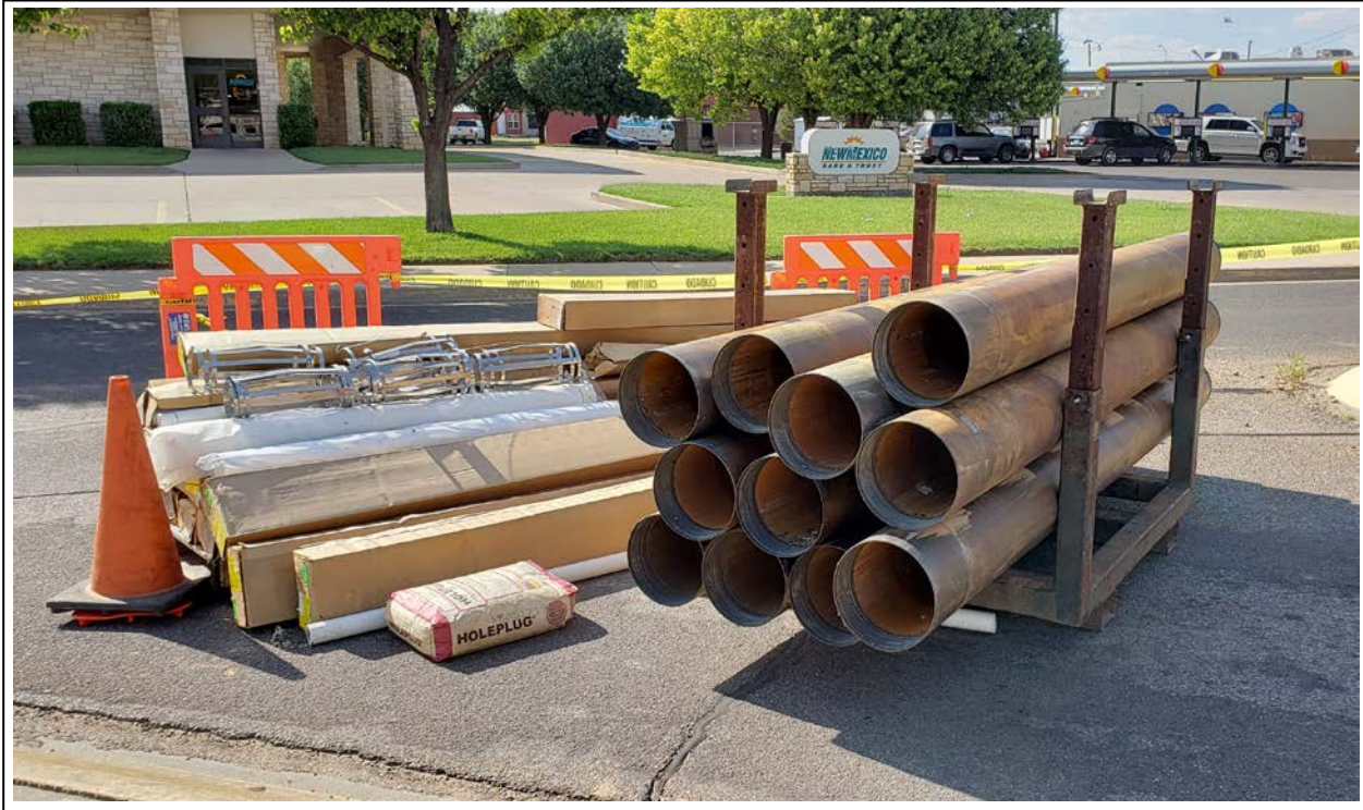
17. Well materials and sonic casing staged in the work zone in the westbound lane of Commerce Way (view to north)
