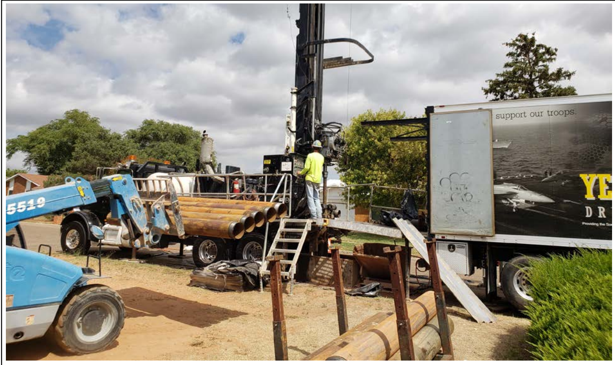
37. Loading sonic casing into the box truck during drilling at MW-14 (view to west)
