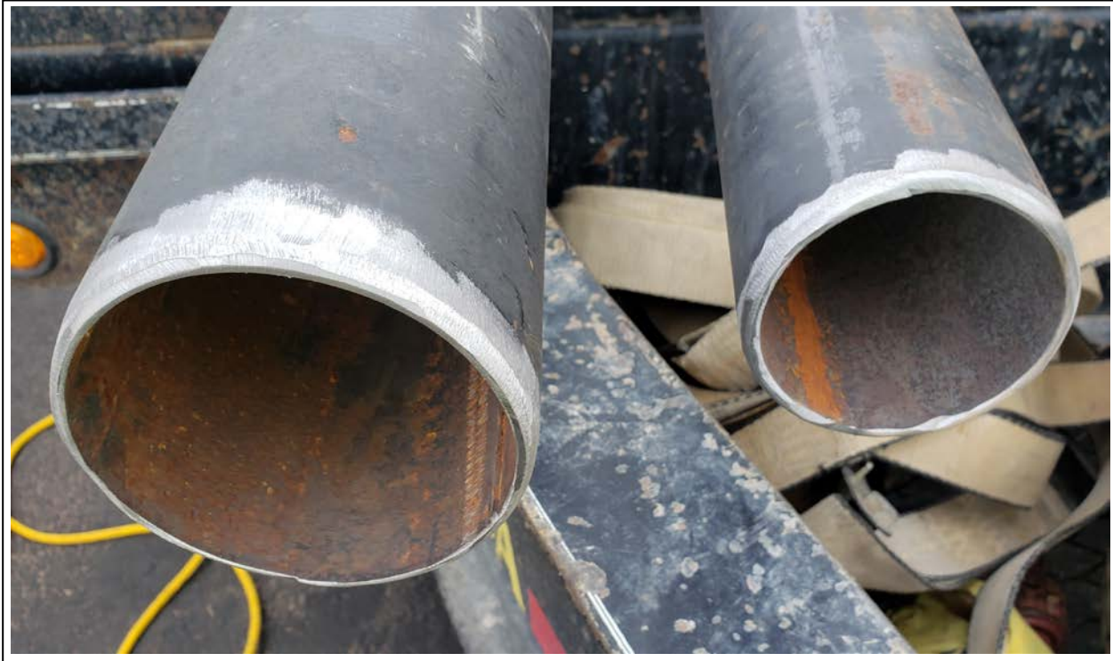
47. Dummies with threads cut off and edges beveled to prevent damage to PVC casing
