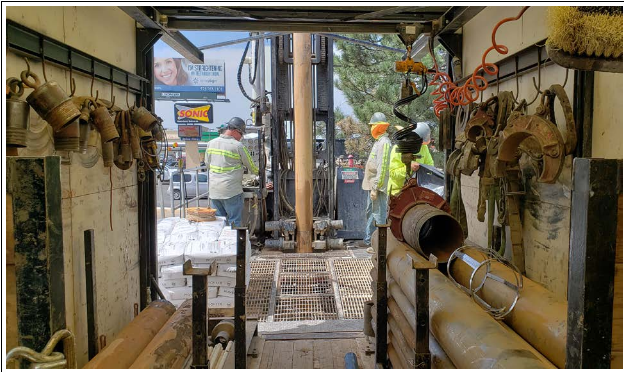
18. Removing sonic casing in preparation for casing installation at RW-1 (view to north)
