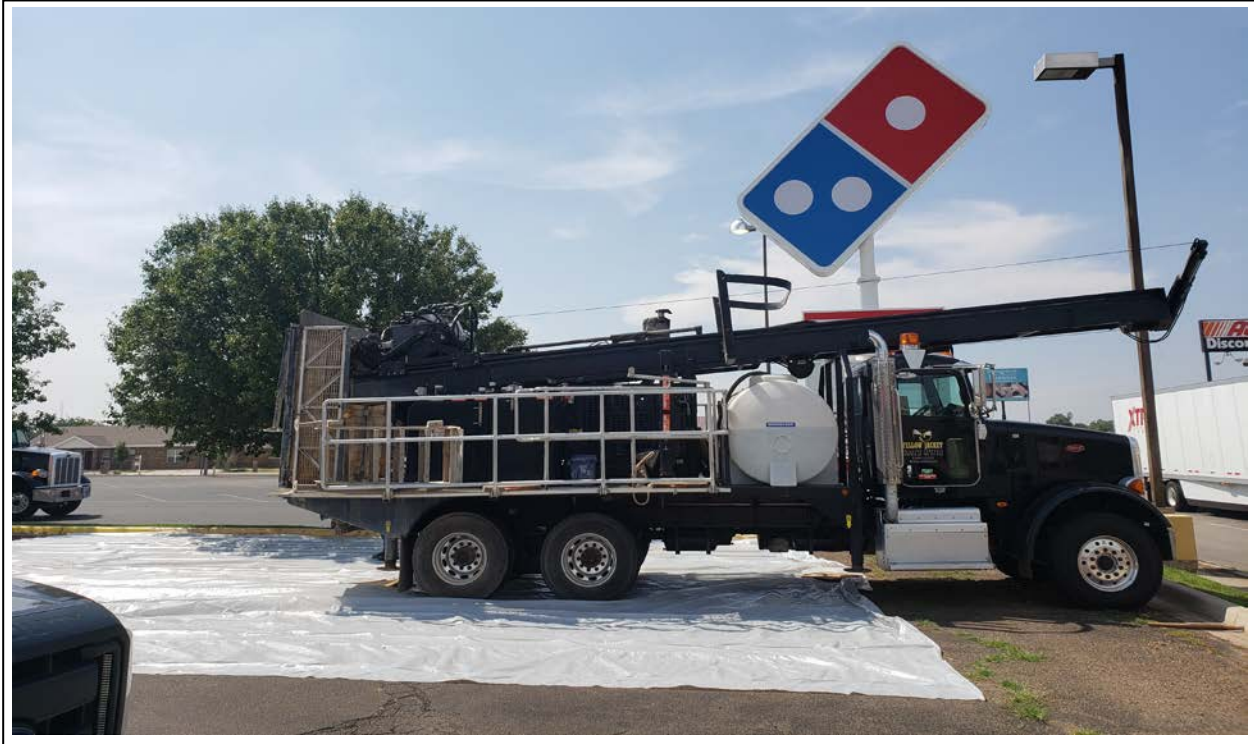
29. Plastic sheeting to contain cuttings and minimize clean-up after drilling is completed at MW-13 (view to south)
