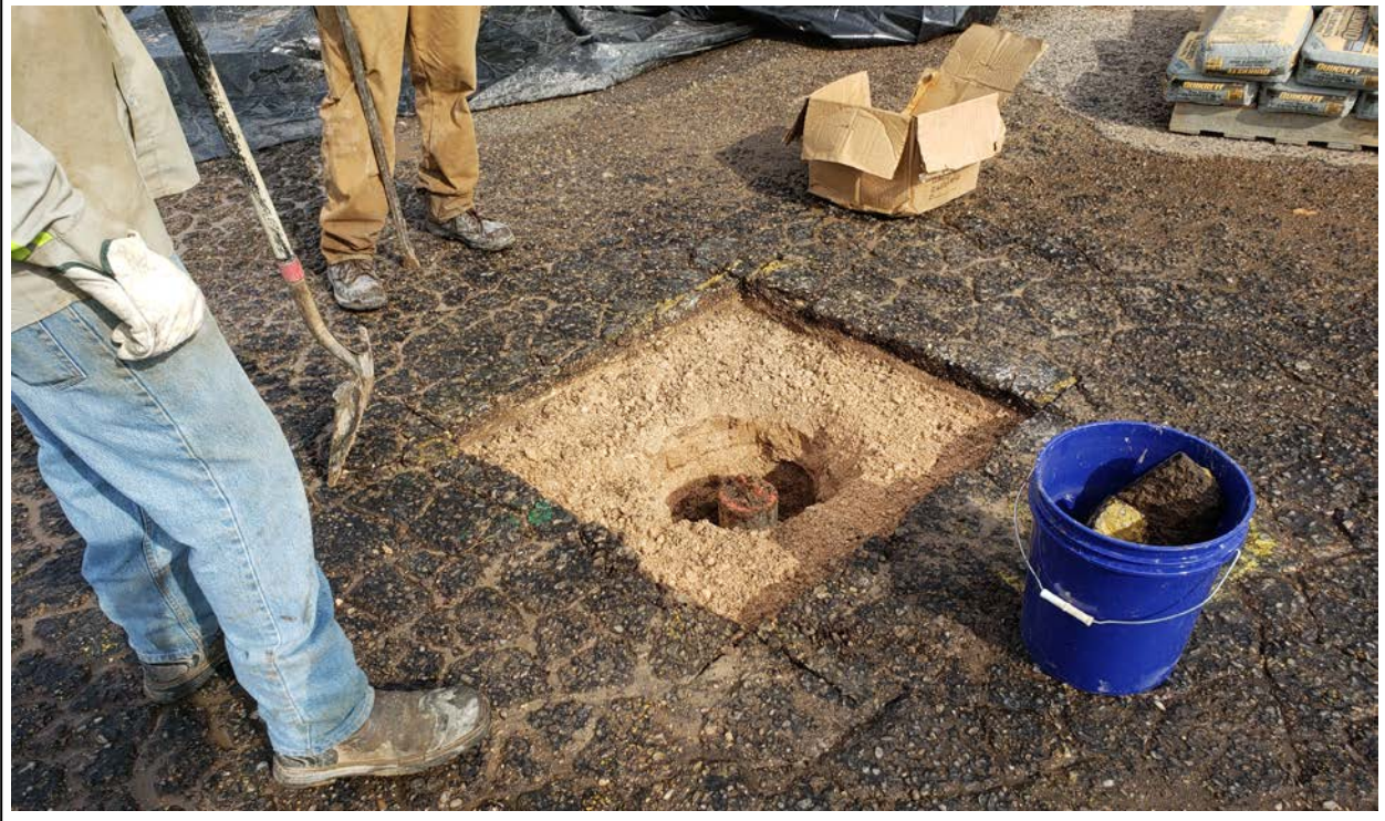
27. Asphalt removed for completion of the well pad at BW-7R (view to northwest)
