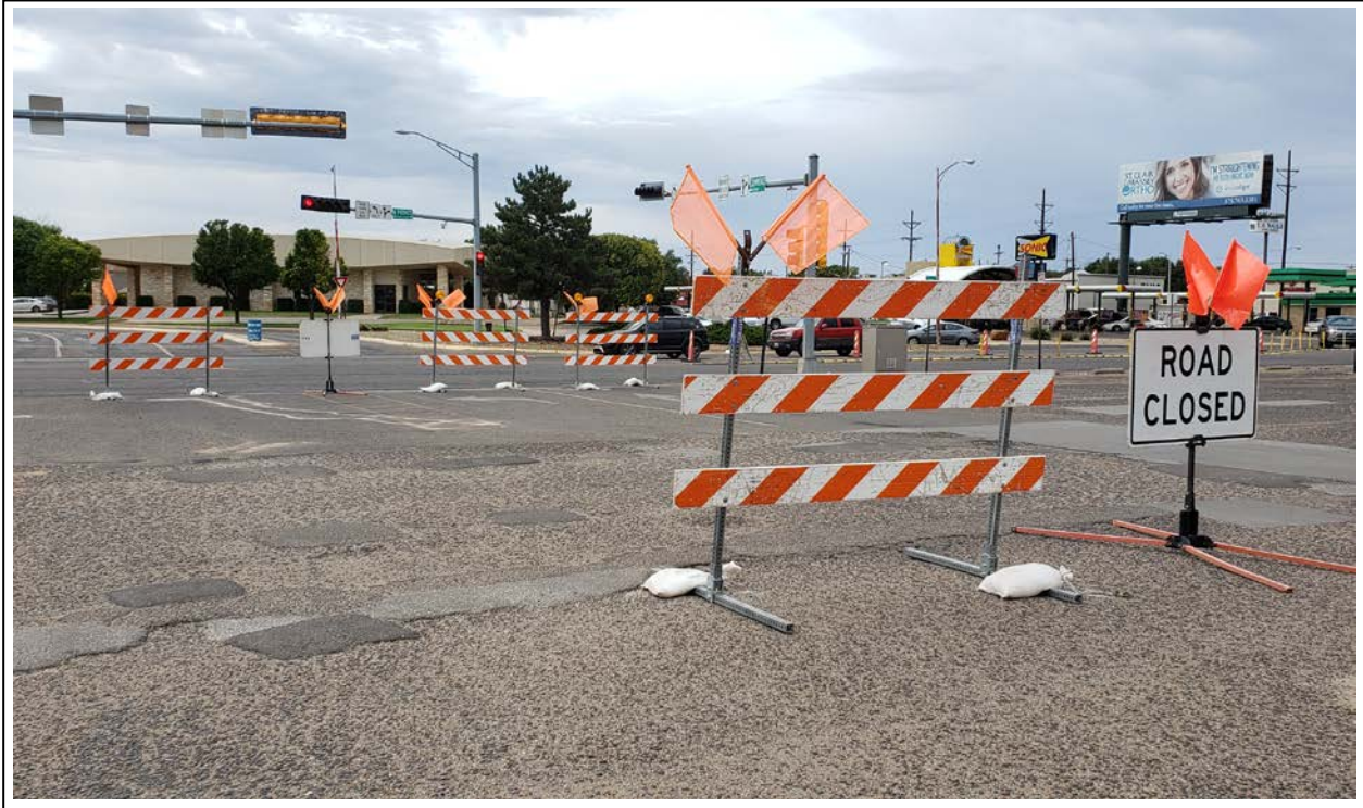
31. Traffic control closing for shopping center entrance across from Commerce Way for installation of RW-3 (view to west)
