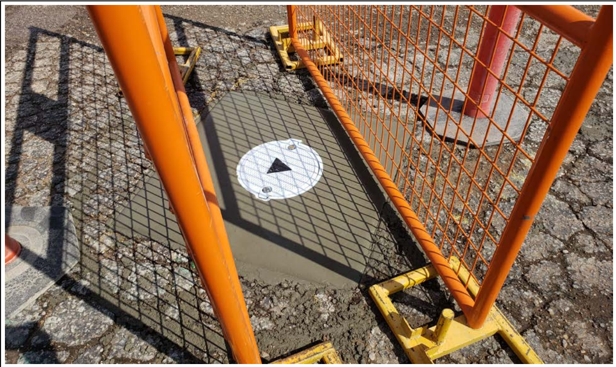
28. Well pad completion at BW-7R with barriers to protect the curing concrete (view to northwest)
