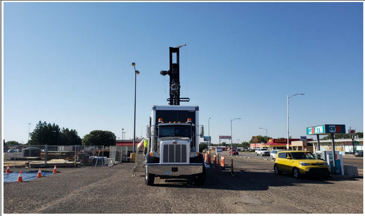
35. Rig and box truck set up for drilling of RW-4, leaving access to the ATM (view to south)
