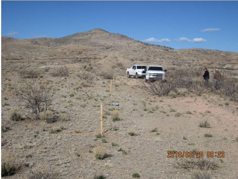
Figure 1: Breach Weir Cross Section Staking along Top of Dike Crest - Looking West (2018-03-28)
