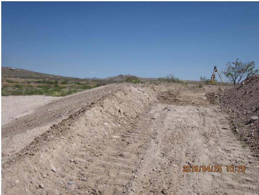
Figure 7: Transit Level East of Weir Breach (2018-04-25)
