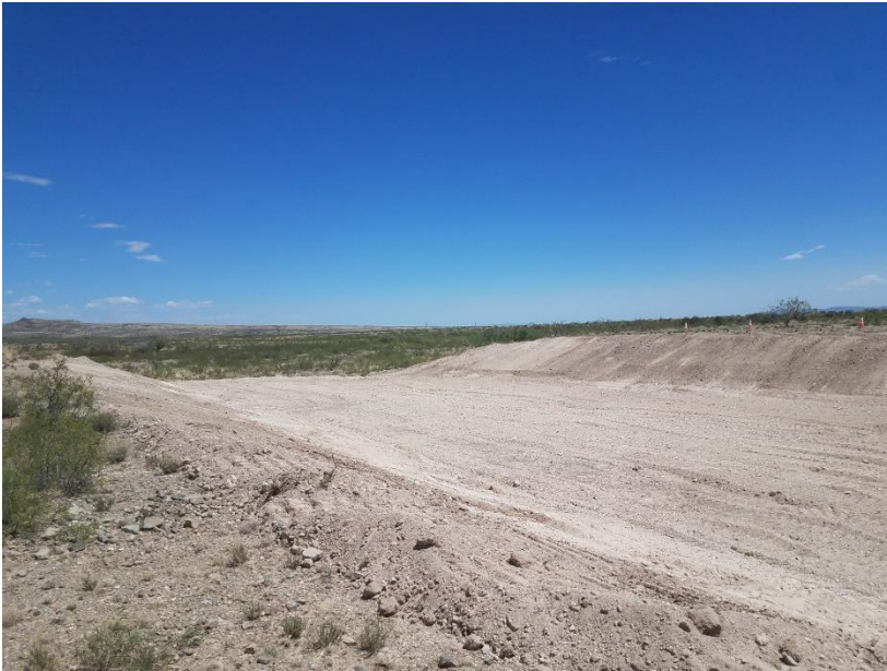
Figure 5: Breach Excavation End (2018-04-23)
