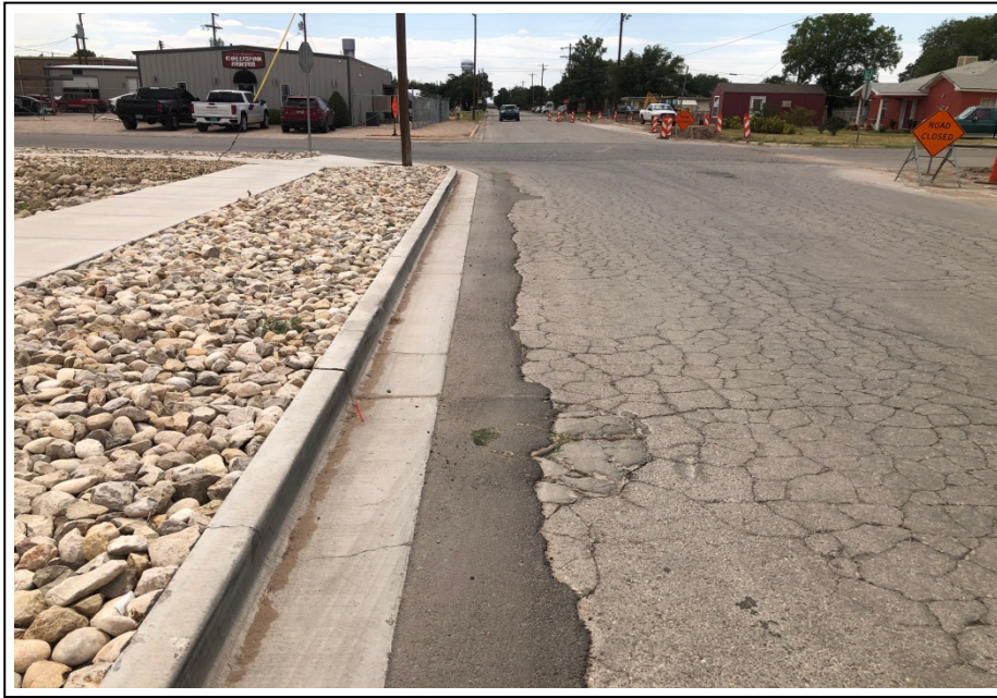
1. Partially paved over well W-7, view to the west.
