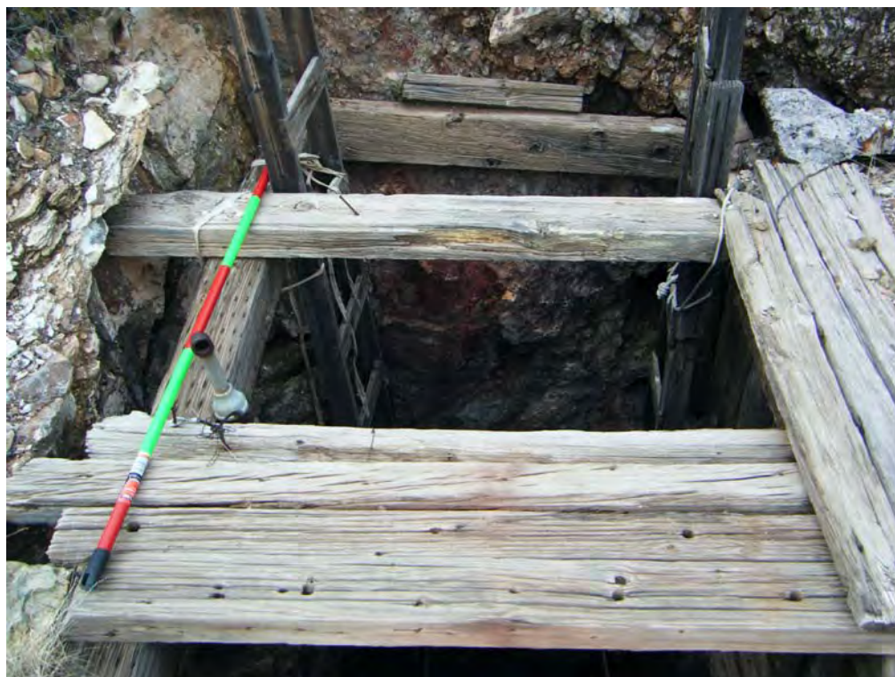
Photo 38– Looking northwest at Shaft-5. Photo (h) in the Anderson report was taken from the opposite side of the shaft.
