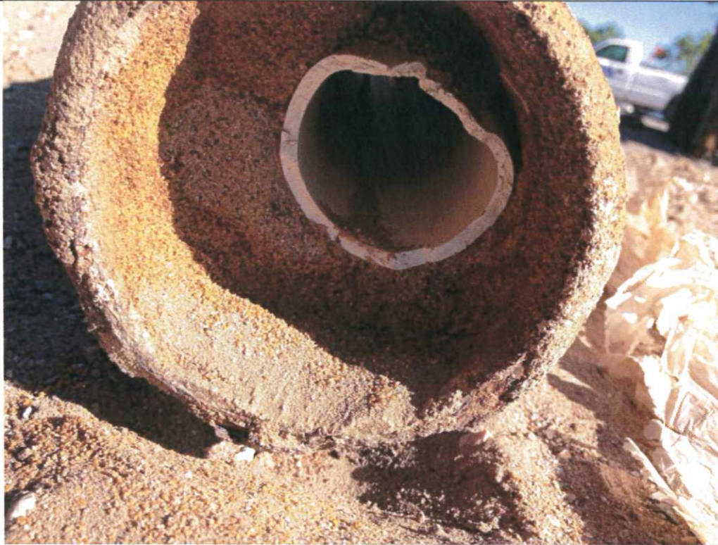
Photograph No. 9 Well MW-4 showing well casing was broken off inside steel casing.
