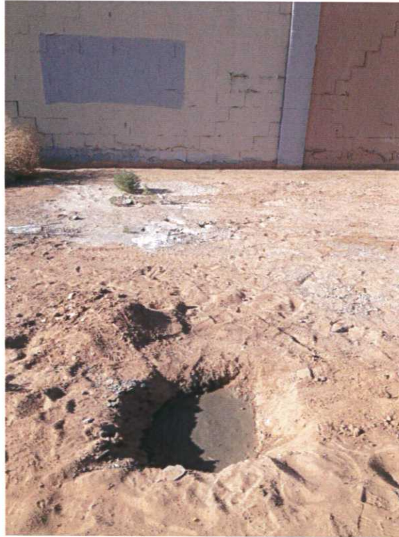
Photograph No. 15 Steel well vault removed and well MW-5 grouted to surface.
