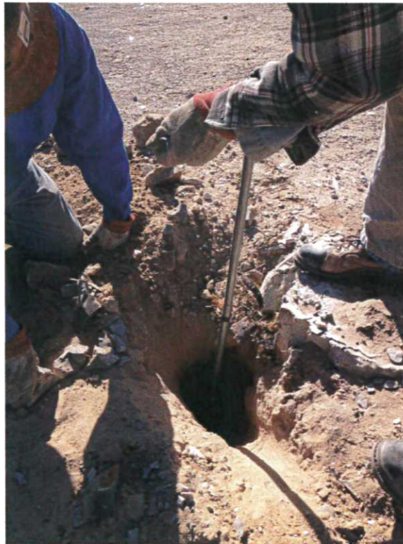
Photograph No. 10 Hand augering to find broken PVC well casing on well MW-4 to abandon.
