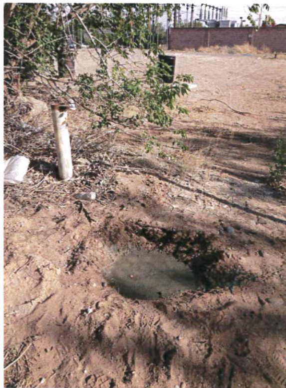
Photograph No. 4 Well MW-1 after removal of steel casing and concrete pad.
