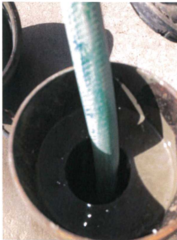
Photograph No. 2 Grouting well MW-1. All wells cement grouted from the bottom up with a pump and a tremmie pipe.
