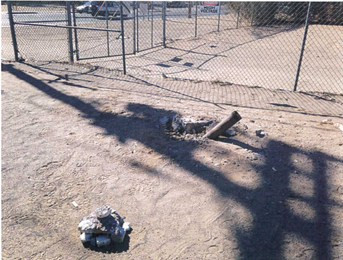
Photograph No. 8 Well MW-4 with bent steel casing (including location of MW-4R marked with cairn).
