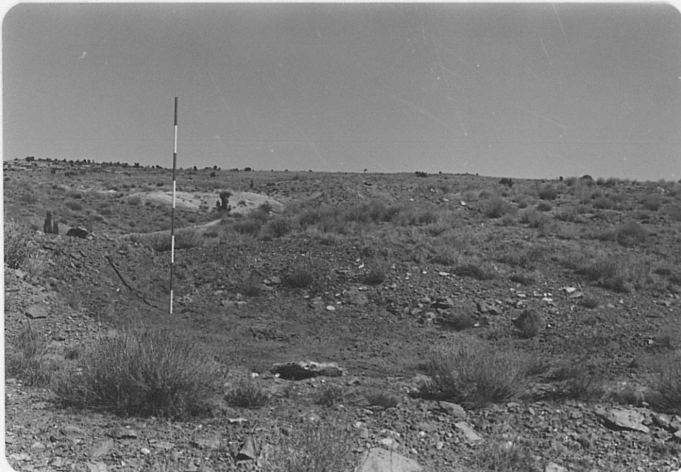
Photo (d) Looking north at small dozer cut with dump from cut in photo (c) visible in background.
