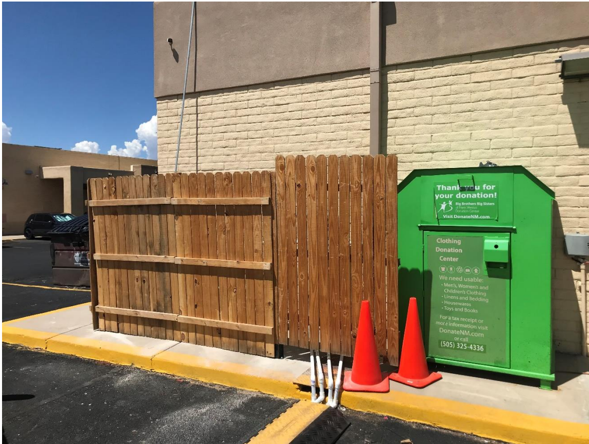
Description: SVE system enclosed in fence.
