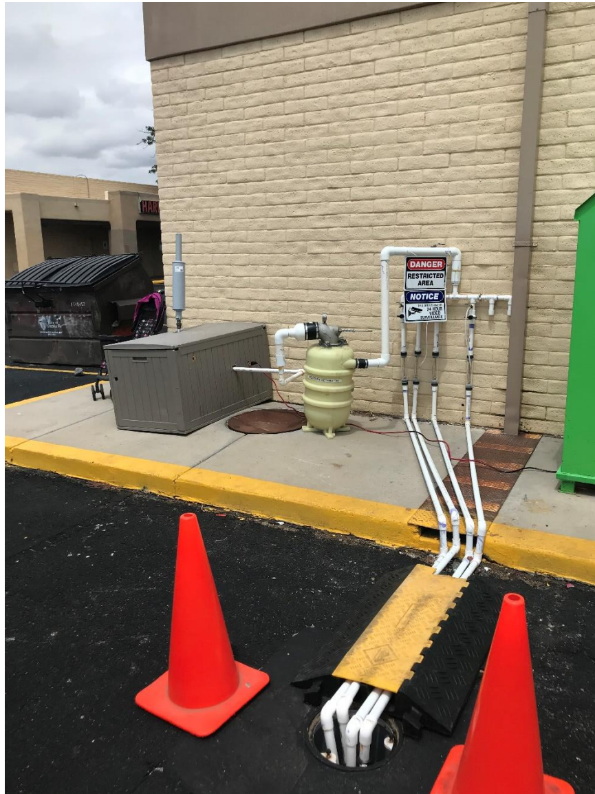
Description: SVE wells plumbed to manifold, knockout pot, and blower.
