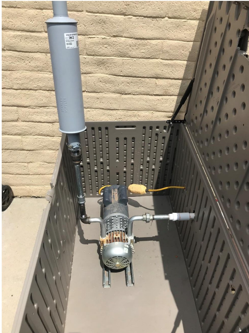
Description: Inside blower box.
