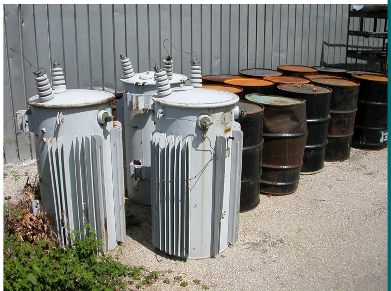
Because of their insulation properties, PCBs were widely used in electrical transformers until they were banned in 1979. PCBs are found at New Mexico orphan sites that handled transformer oil as well as old landfills.
