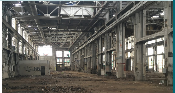
In addition to environmental and human health risks, orphan sites can present significant safety risks due to the presence of abandoned structures, deteriorated equipment, and open foundations.
