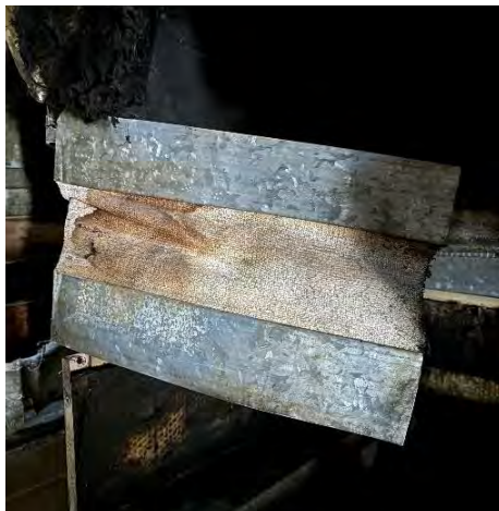
Heater Duct Flex Joint
