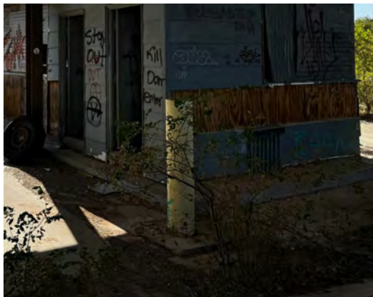
All Exterior Lead-Based Painted Lower Walls
