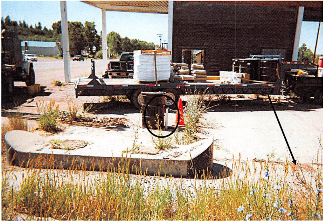
No. 1 – View looking south at MW-1 (circled) prior to completion. Note abandoned pump island in the foreground and existing petroleum tank vault (arrow).
