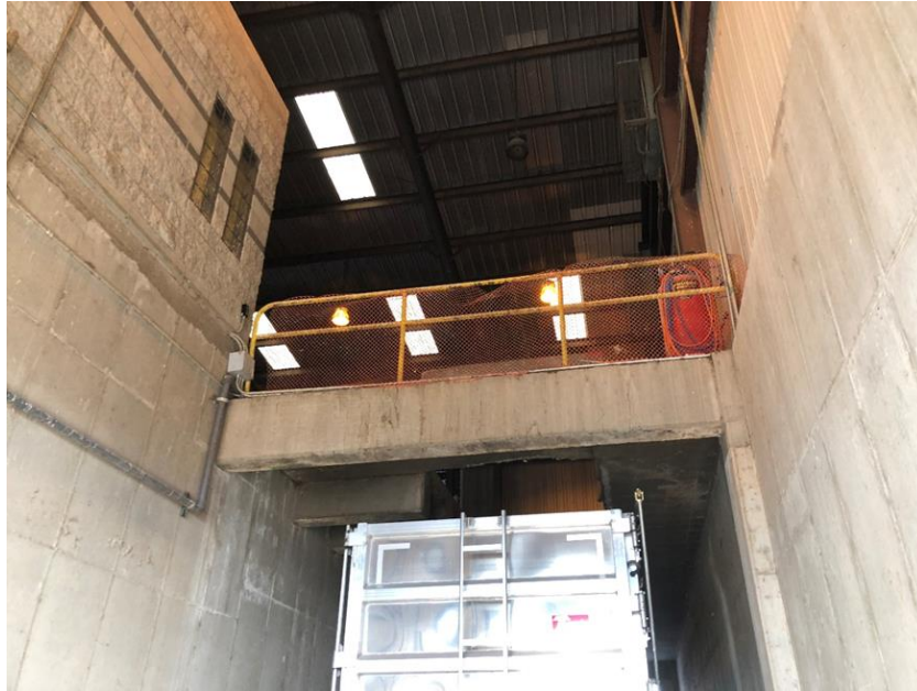
FIGURE 6-1 LOWER LEVEL OF TIPPING FLOOR AND COLLECTION TRUCK
