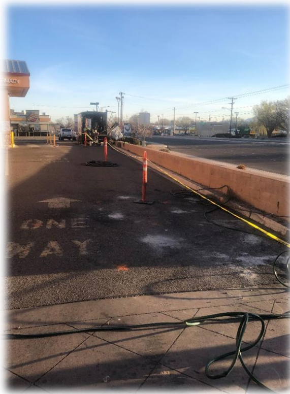
View of MW-08 injection area
