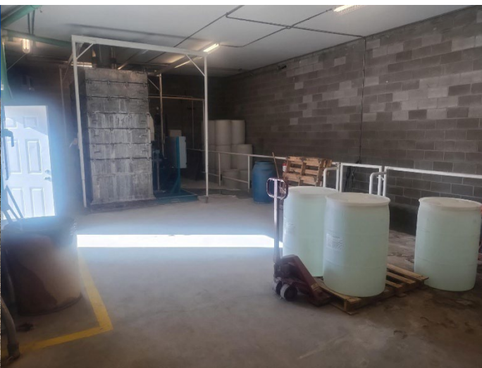
CW-1 Pump house interior with aquamag drums
