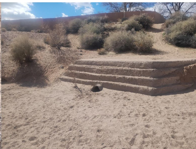
CW-1 Infiltration Gallery Looking South
