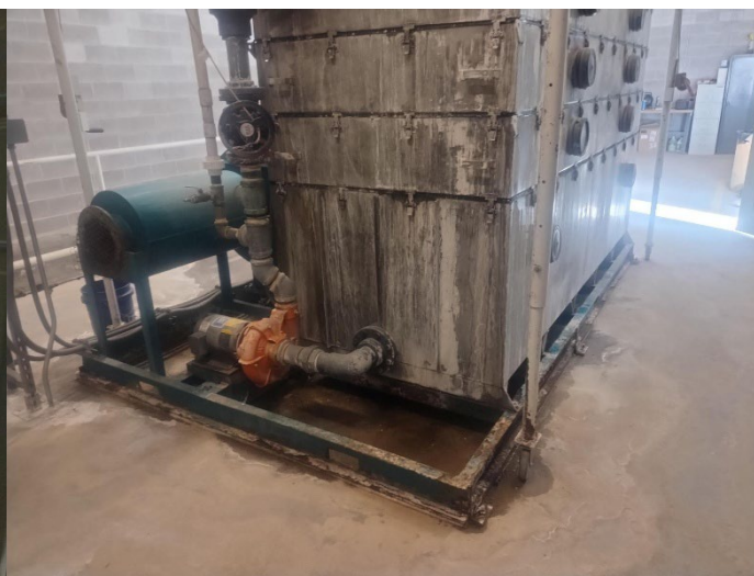
CW-1 Air Stripper
