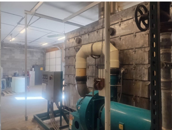
CW-1 Air Stripper
