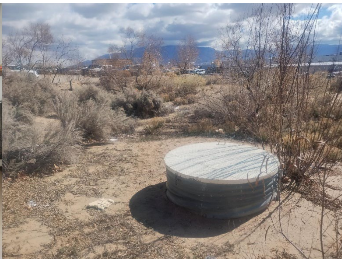
CW-2 Well vault
