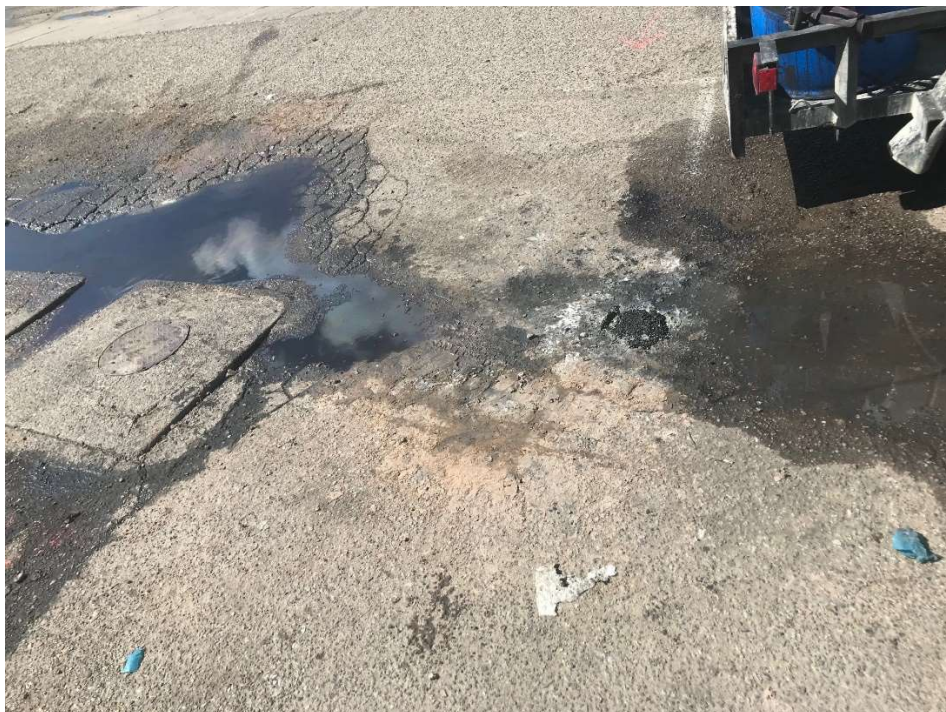
Borehole Patched with Asphalt
