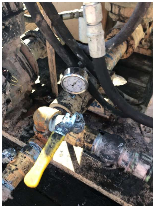
Injection Pump, Pressure Gauge, and Shut-Off Valve
