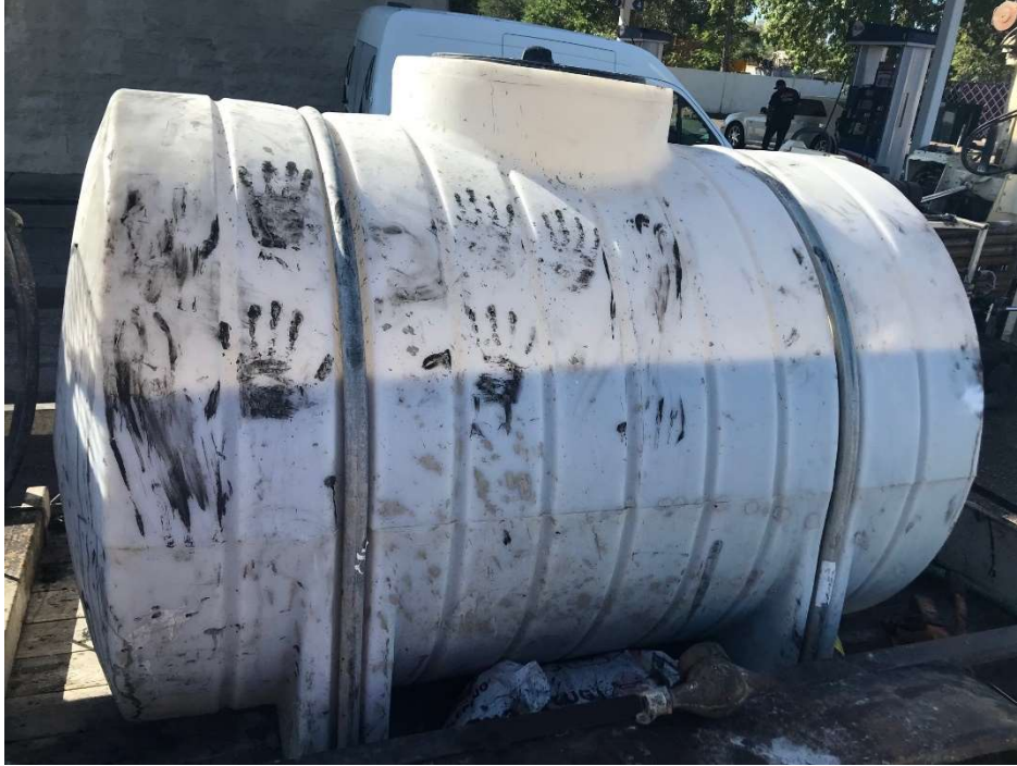
Water Holding Tank
