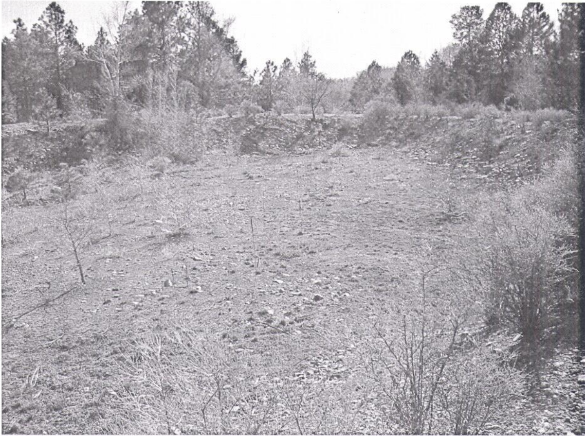
Excavated area that would be used to develop the second pond at Eagle Rock Lake
