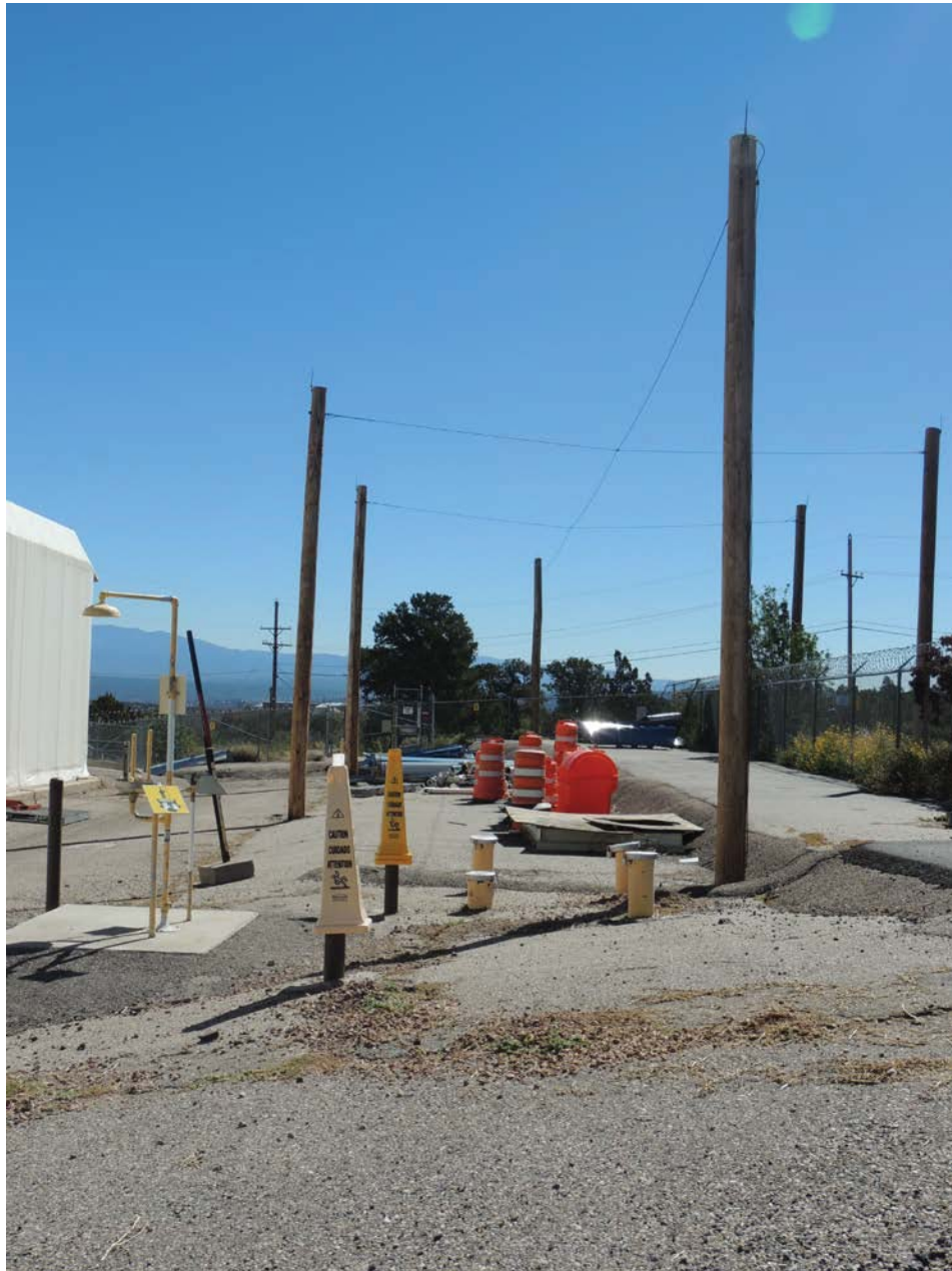
TA-54, Area L, Process Code D80, Disposal Shafts 13-17 and 19-28 (To be closed)
