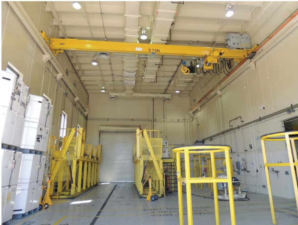
TA-54-38 West Indoor, High Bay, Process Code S01, Container Storage Unit
