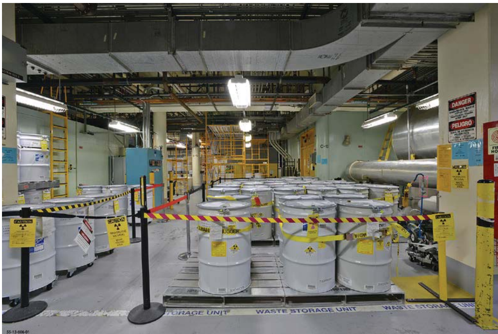
TA-55-4, Basement, Process Code S01, Container Storage Unit (B40) (View is looking southwest)
