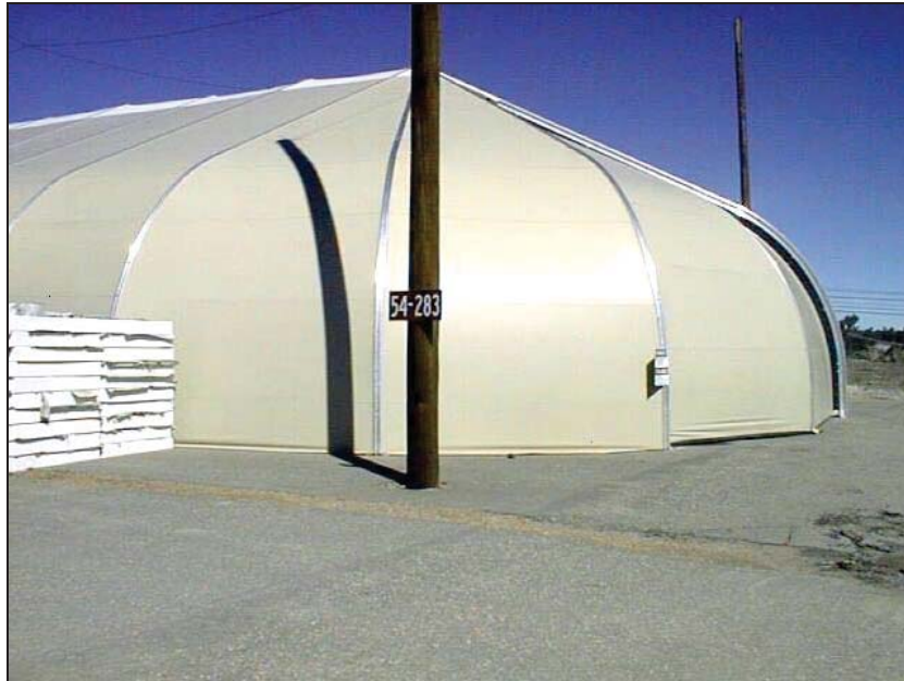
TA-54-283, Area G, Storage Dome Process Code S01, Container Storage (Pad No. 6)
