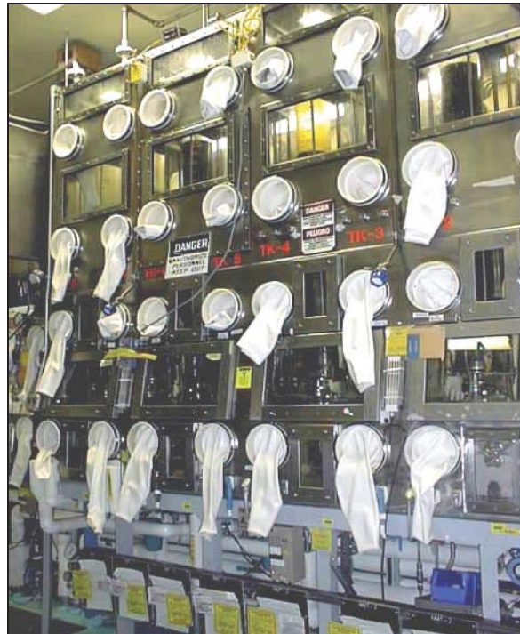
TA-55-4, Room 401, Evaporator Glovebox Tanks Component Process Code S02, Storage Tank System
