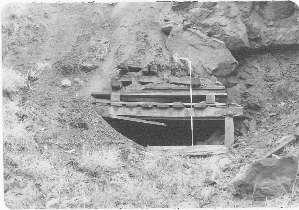
Photo (e) Close up of decline show in photo (d); present opening is less than 3' high. Note range pole for scale.
