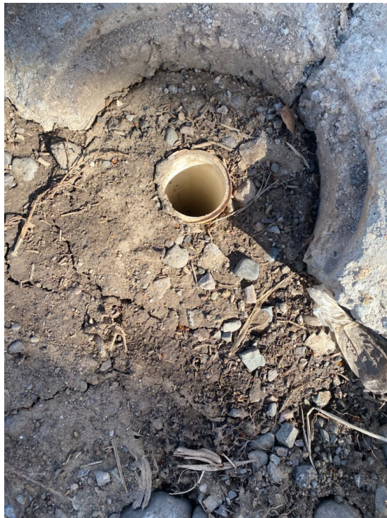
MW-12 vault missing
