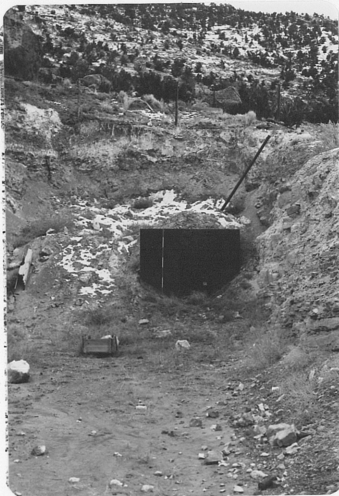
Photo (f) Close-up of sec. 34 portal; note range pole in front of metal door for scale.
