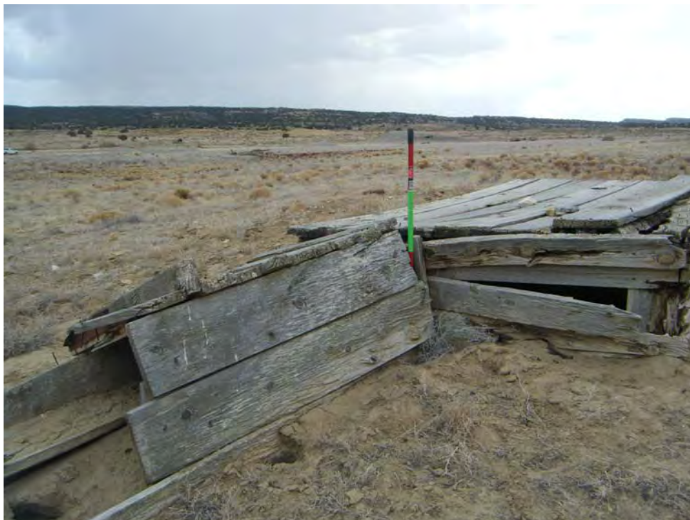
Photo 20-Looking west at StructPly-2, referred to as a “powder magazine” in the Anderson Report.
