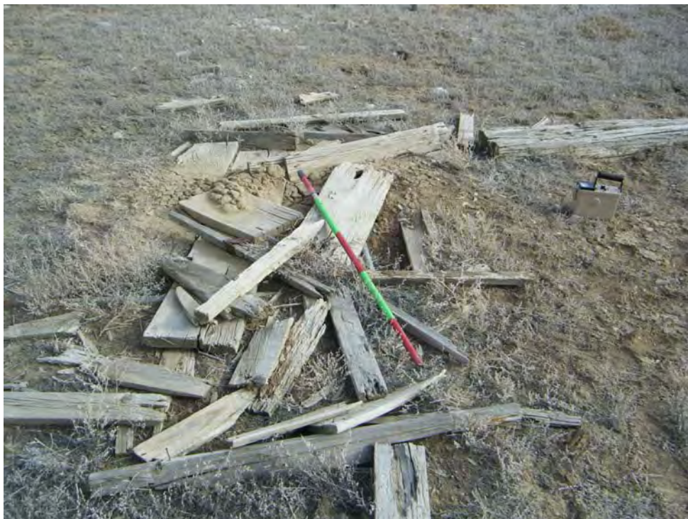
Photo 26-Looking south at collapsed structure (StructPly-3).
