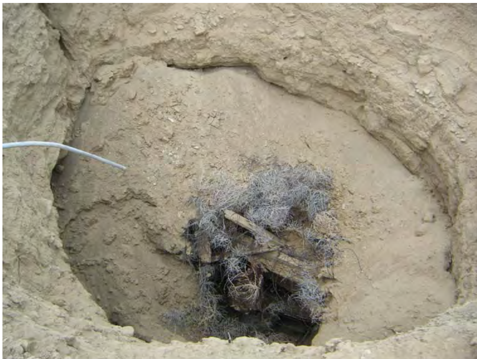
Photo 18-Looking down into ShaftPly-1, caved depth was approximately 50 feet or more (note timber in center of shaft).
