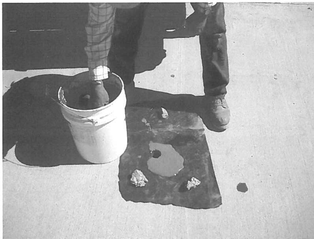
Photograph 3. Pouring neat cement grout into MW-1; keeping grout off of pavement using small piece of visqueen liner with a 2-inch diameter hole placed over the well casing.
