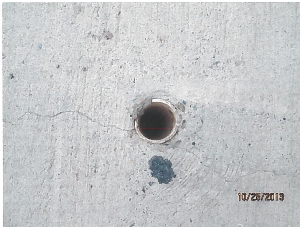
Photograph 2. Close up of MW-1 showing how concrete was poured around casing during concrete pavement construction in 2000.
