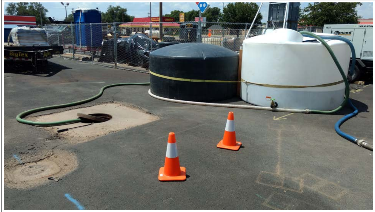
3. Treated effluent discharge to city sewer
