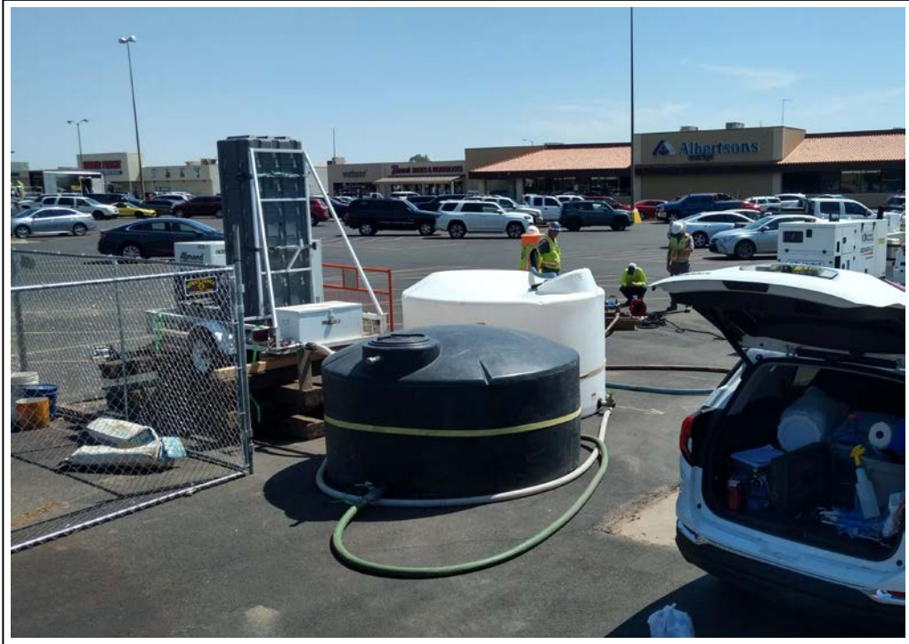
1. Site setup: primary and secondary discharge holding tanks in the foreground adjacent to air stripper tower, with pumping well behind (view to the northeast)
