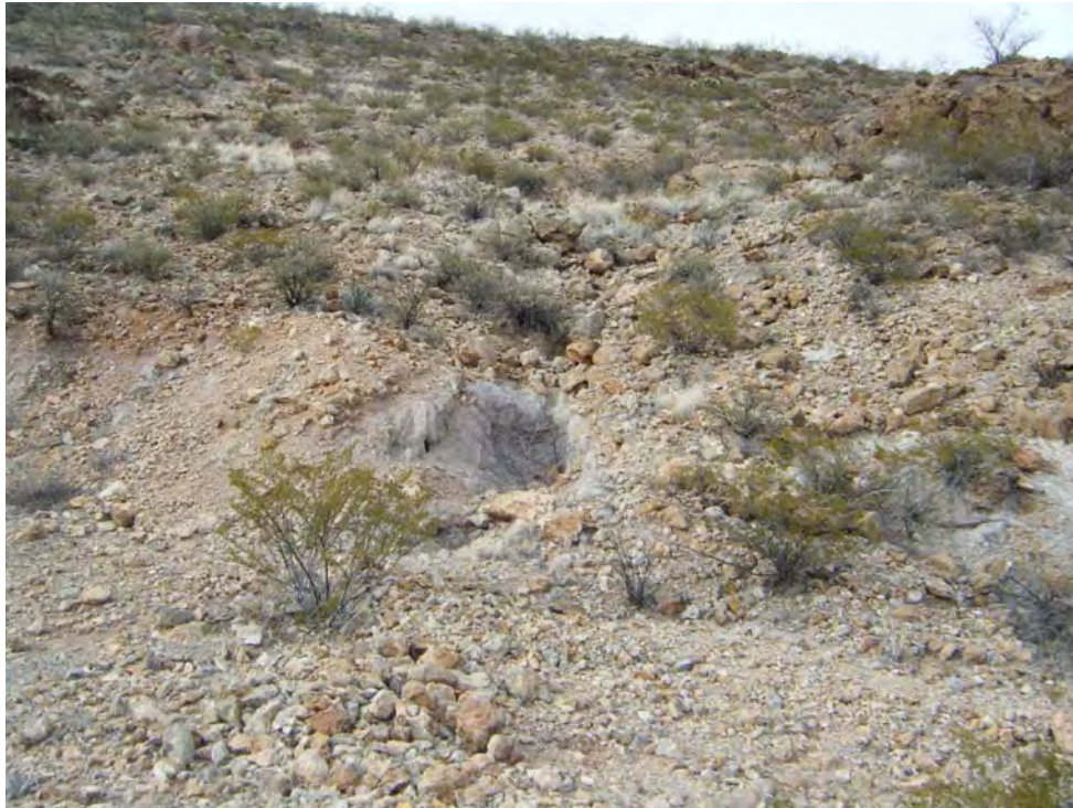
Photo 4 – View of road (rd-1) in foreground and erosion (erospt-1) on slope southeast of the AUM Site, looking north.
