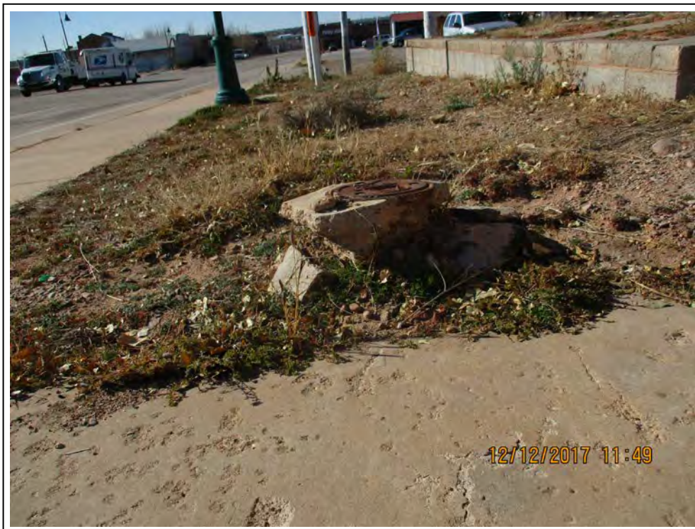
2. Monitor well MW-3 prior to replacement of surface completion (view to the southwest).
