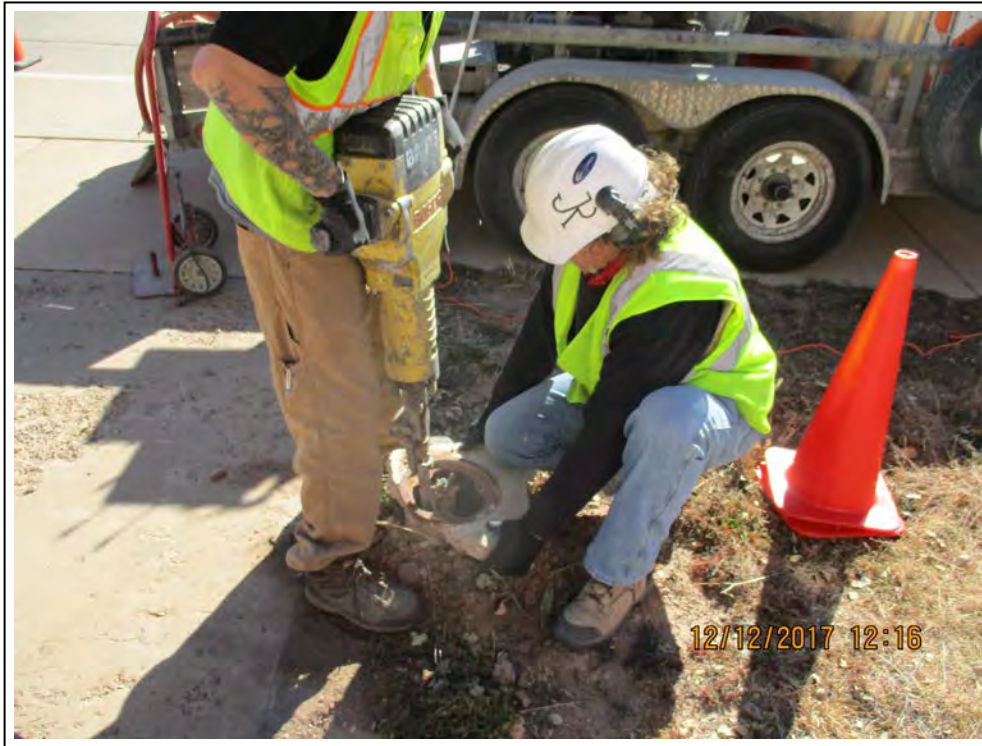
3. Breaking up concrete pad and removing well vault (view to the southeast).
