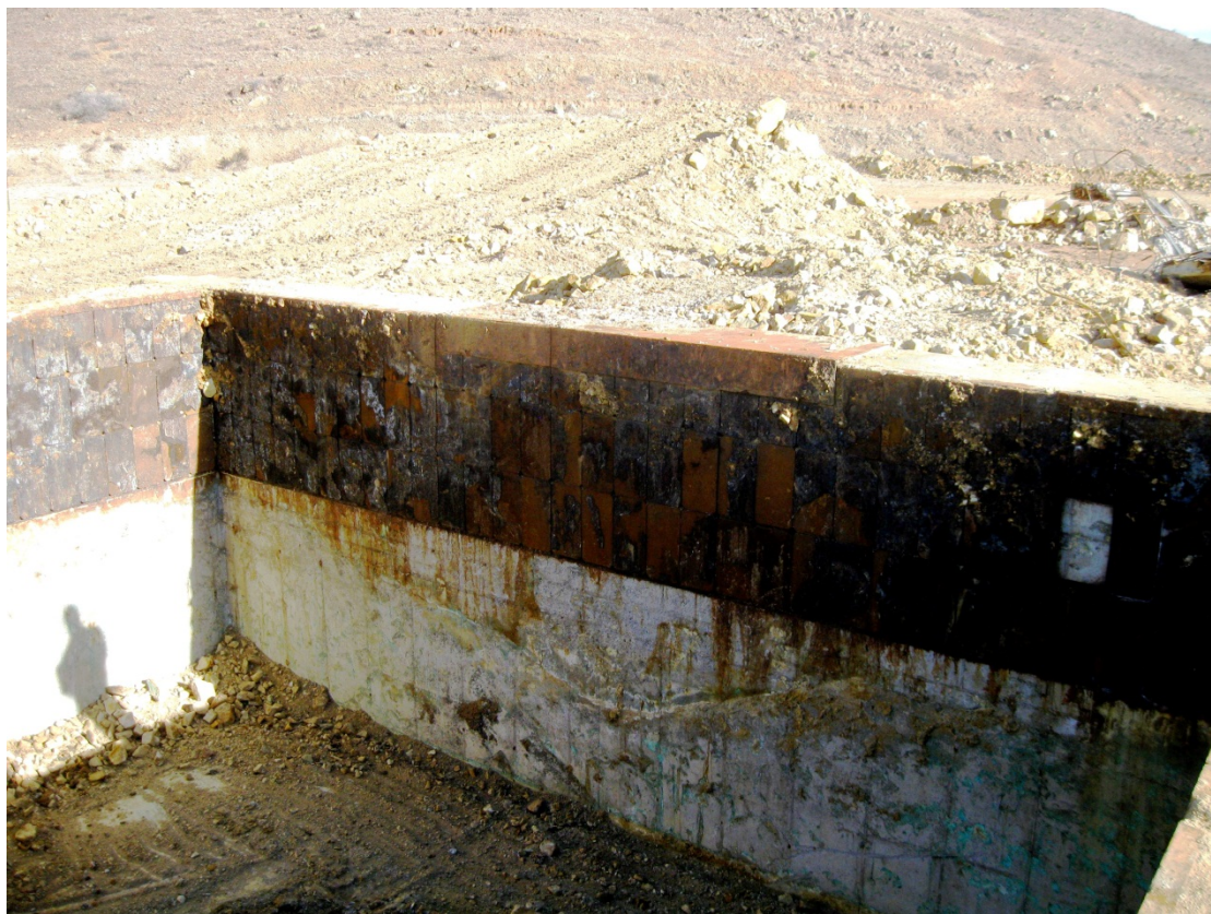
Photo 3 – Primary Crusher – Greenish-blue Discoloration at Wall Surface
