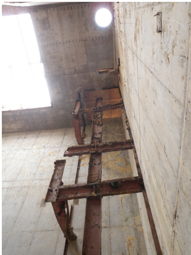
Photo 6 – Primary Crusher –Remains of Elevator Structural Steel
