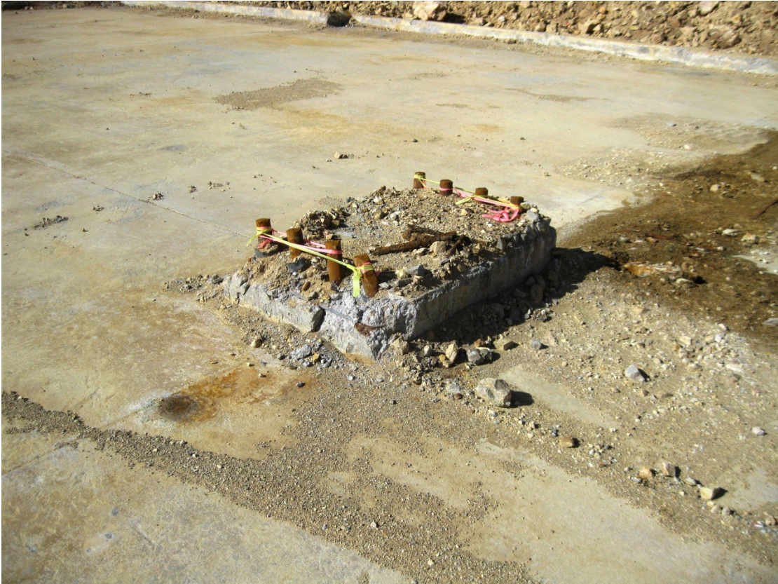
Photo 13 – Truck Shop – Spalled Concrete, Exposed Rebar and Corroded Anchors at Interior Concrete Pier
