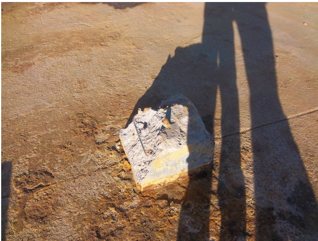
Photo 9 – Flotation Area – Spalled Concrete with Exposed Rebar and Corroded Anchor
