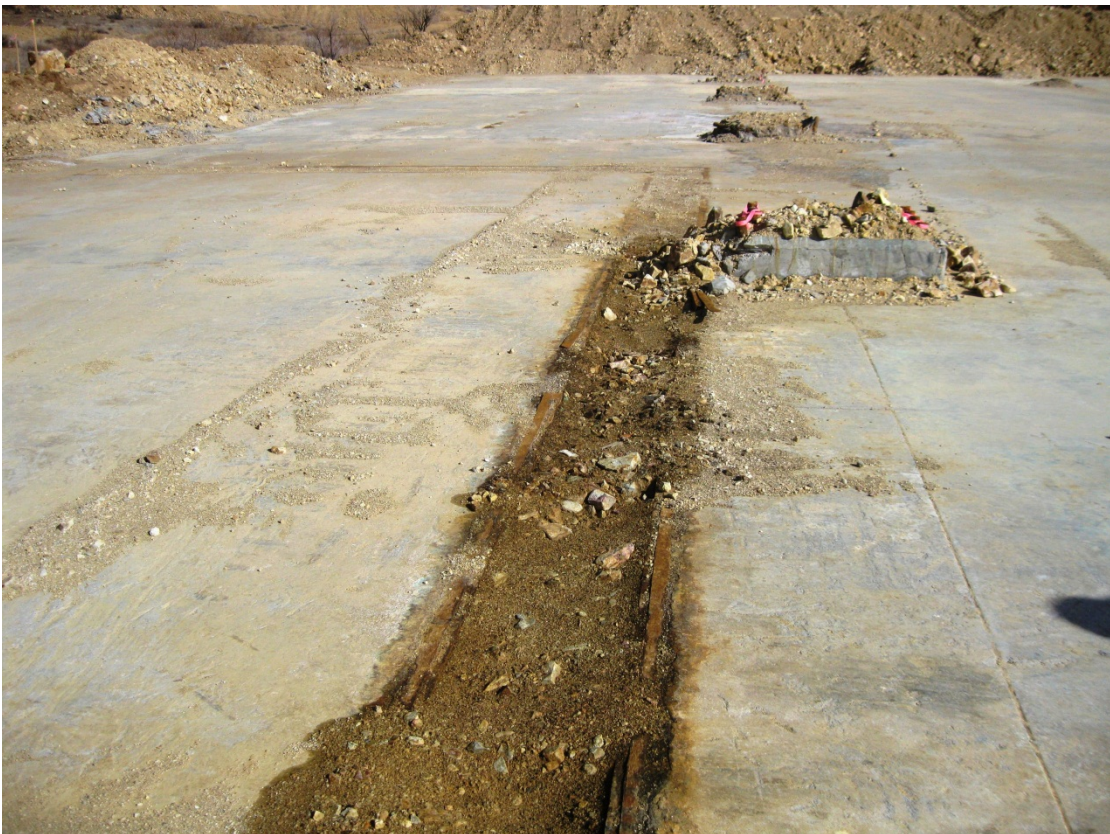
Photo 14 – Truck Shop – Corroded Electrical Trench Embed Angle
