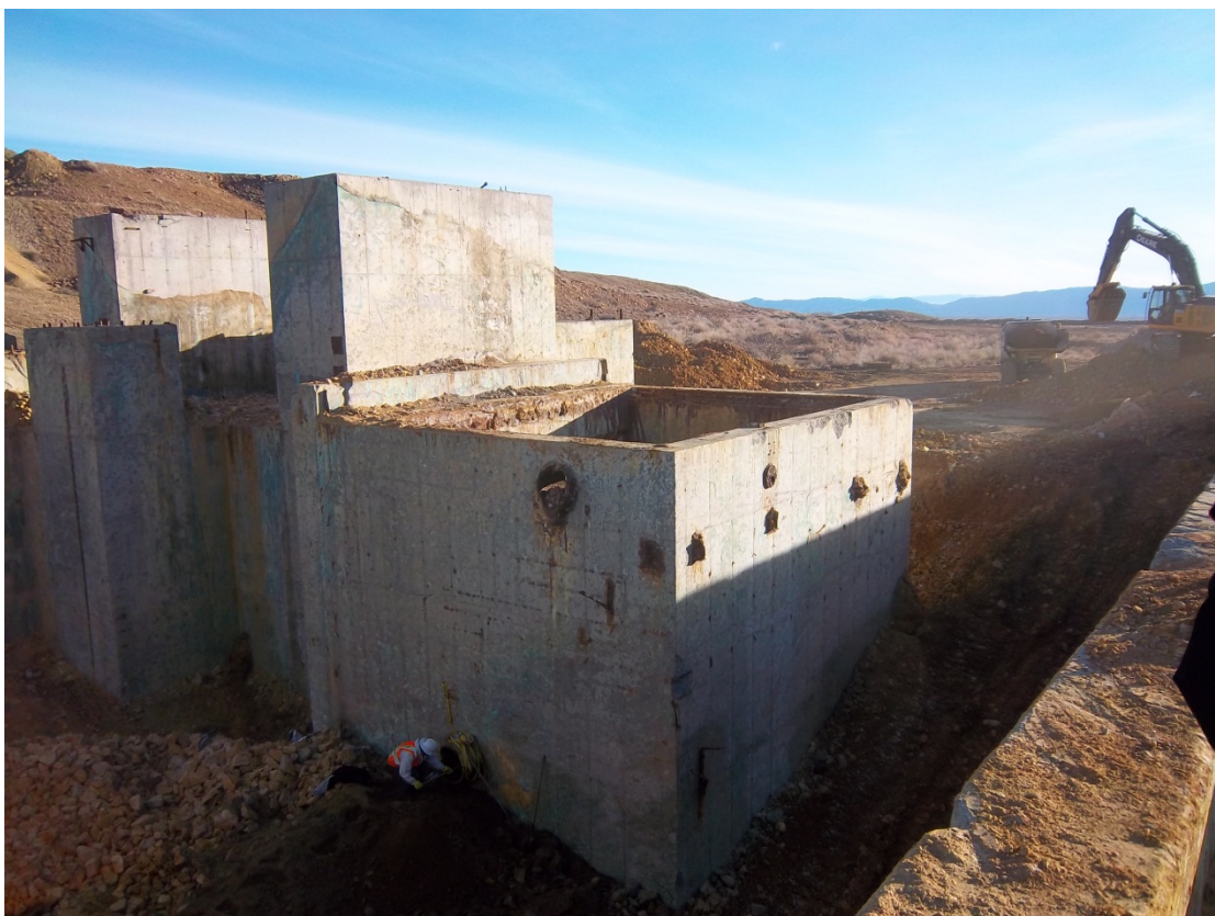
Photo 10 – Grinding Area – Corroded Embeds at Sump Box
