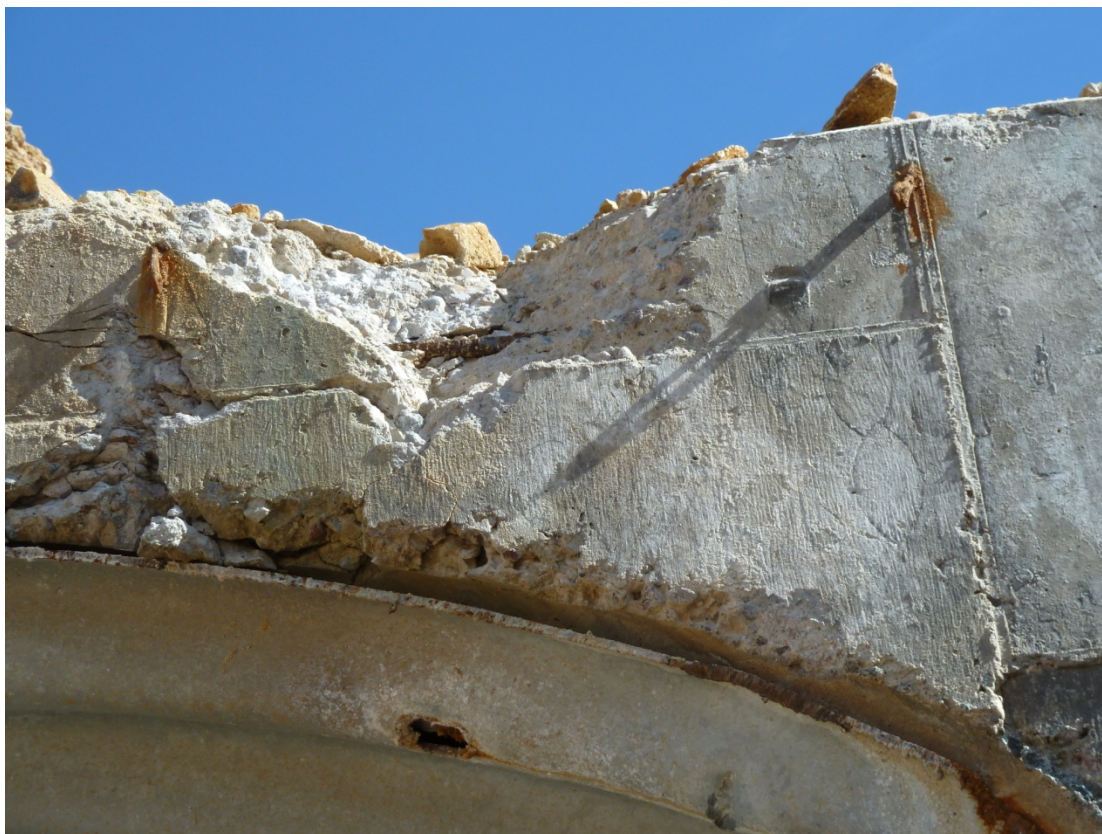
Photo 2 – Damage at Top of Tunnel Entrance
