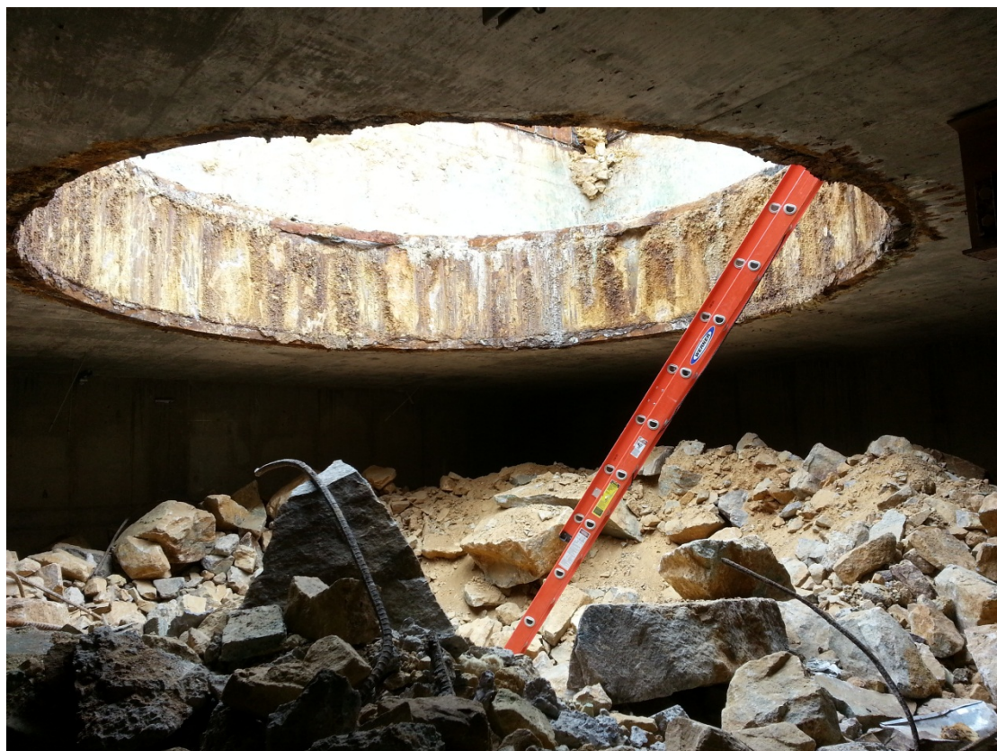
Photo 4 – Primary Crusher – Corrosion on Embedded Items
