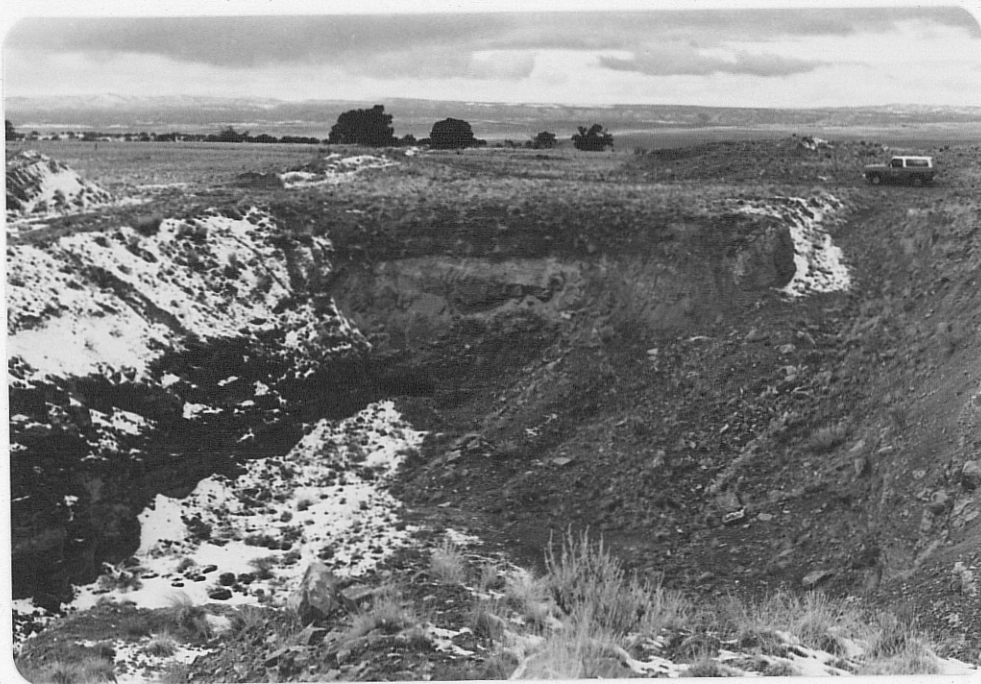
Photo (b) Looking westward at box cut; note ramp at upper right.
