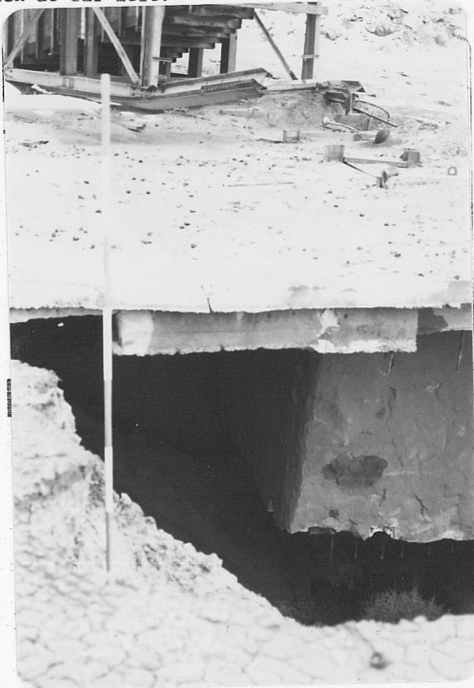
Photo (d) Close up of concrete slab over mine shaft showing void beneath; note range pole in foreground and again the ore bin.
