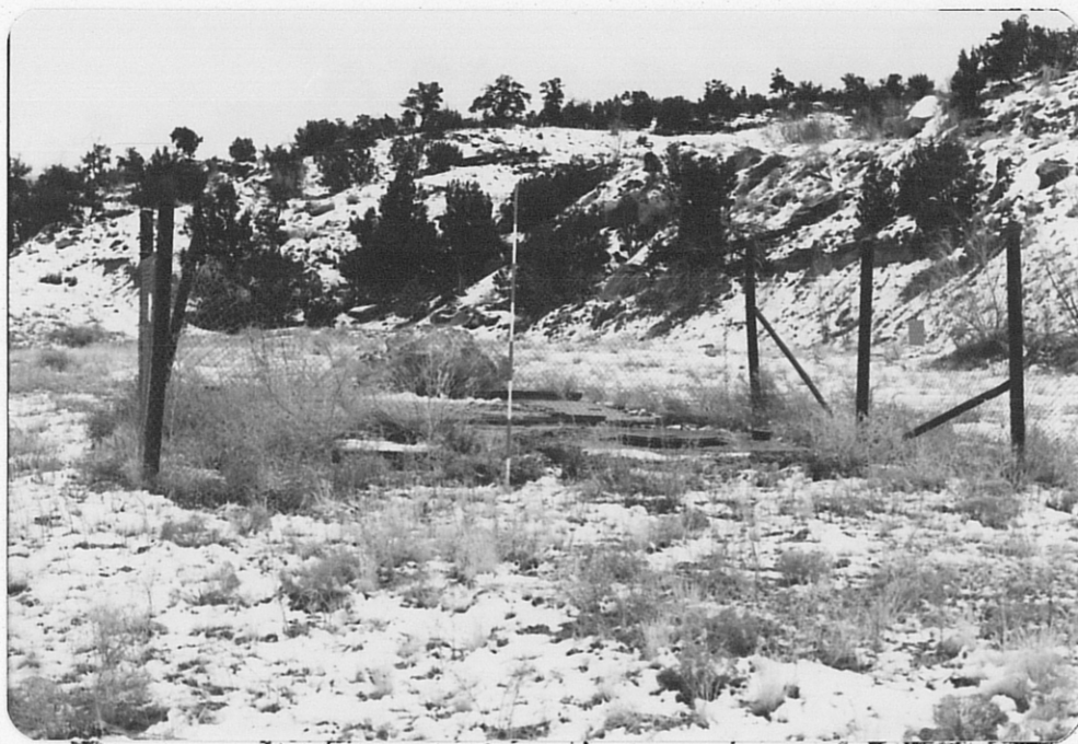
Photo (e) Looking eastward at 30" diam. ventillation shaft and foundation for blower motor. Wire mesh fence surrounding site has been partially destroyed.
