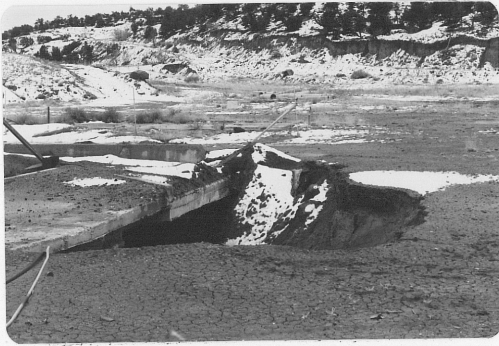
Photo (c) Close-up of shaft site showing extent of caving; concrete slab is 8" thick at far left.
