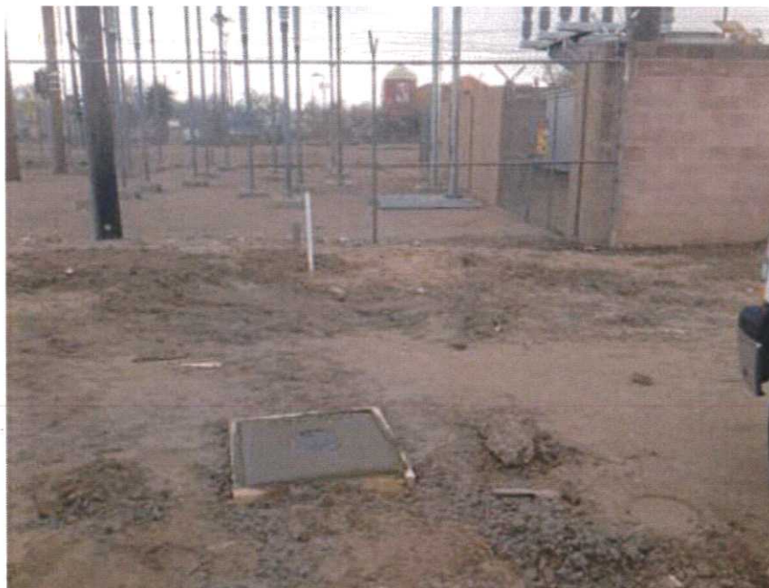
Photograph No. 22 Well vault and concrete pad for newly installed MW-6RR, looking south.
