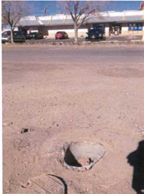
Photograph No. 7 View of NMW-1 with lid removed from vault.
