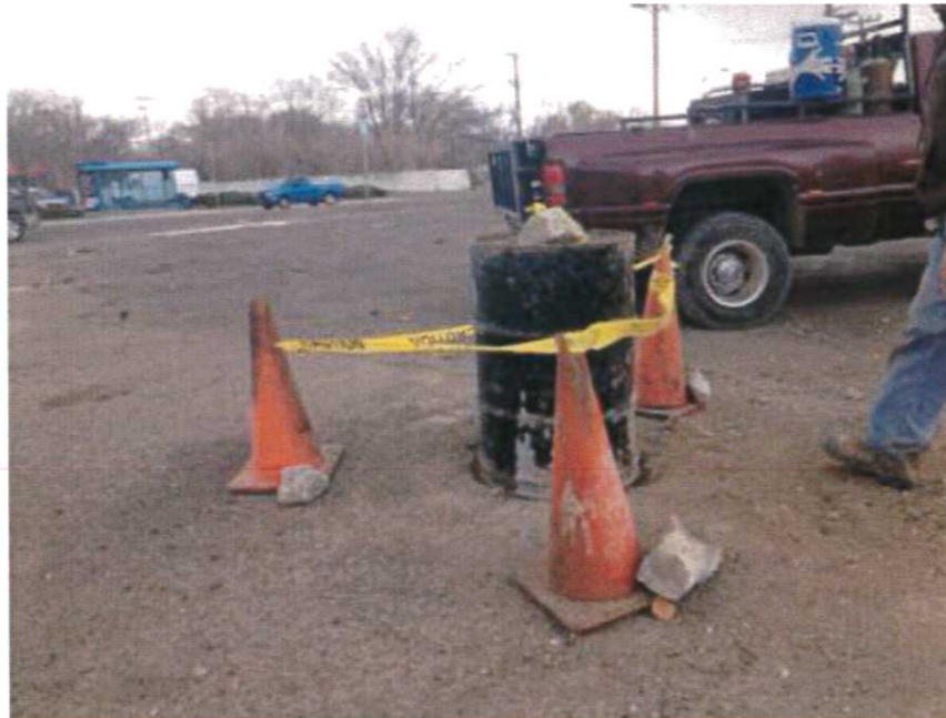
Photograph No. 10 Well vault and pad secured prior to leaving the site to allow concrete to cure.
