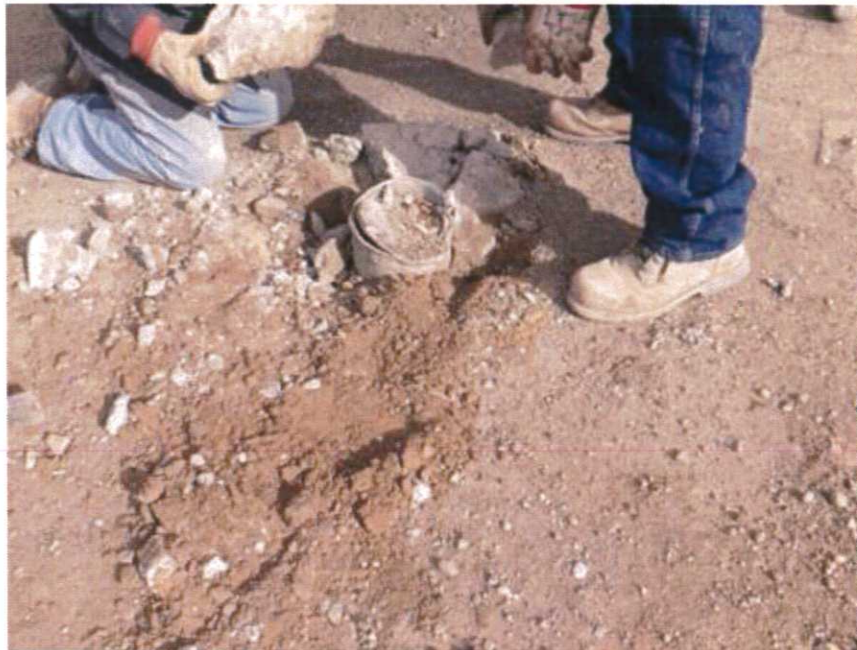
Photograph No. 8 Repair activities for NMW-1. Old concrete well pad and well vault were removed.
