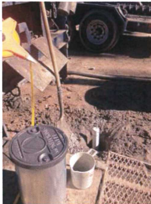
Photograph No. 20 Newly installed replacement for MW-6R, MW-6RR, with bentonite pellets hydrating.
