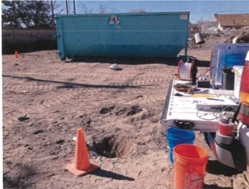
Photograph No. 11 Missing well vault for RNMW-2.
