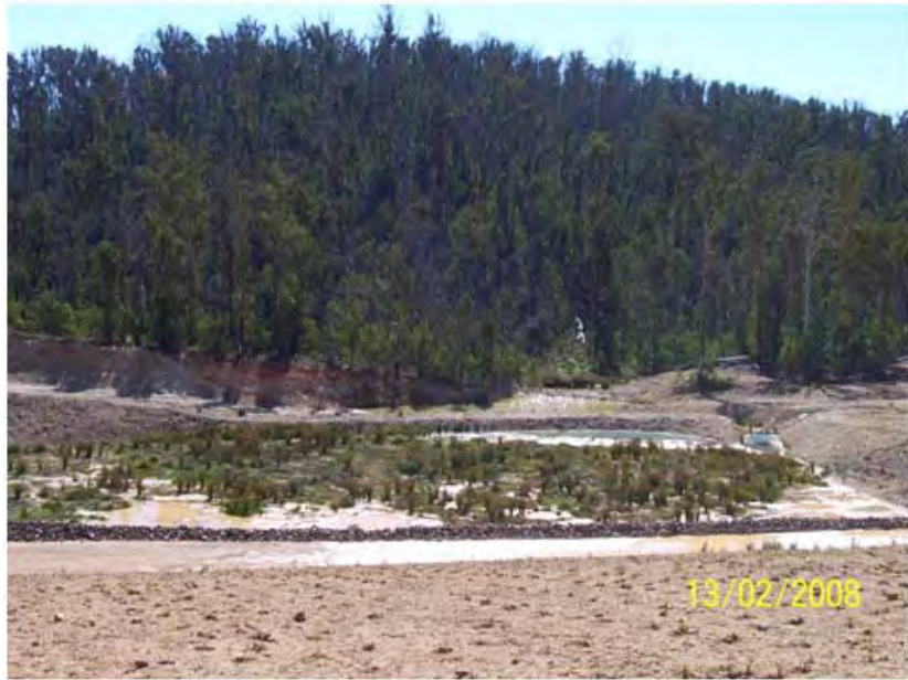
Plate 2. View of the vertical upflow anaerobic wetland that was constructed for passive treatment
