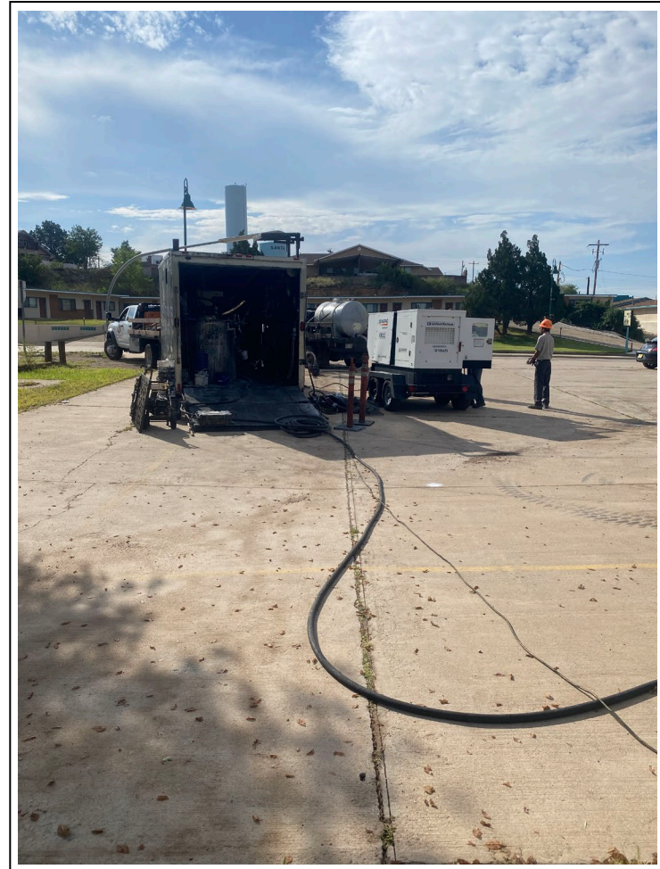
2. Vista's injection truck and trailer (view to south)
